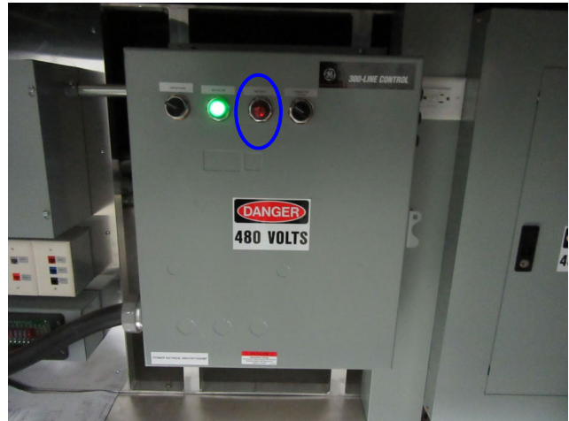
Figure 50: 480V AC Fault Indicator Light
