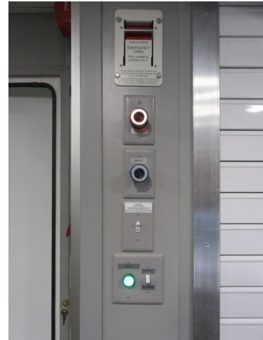
Staff Entry Door Controls
