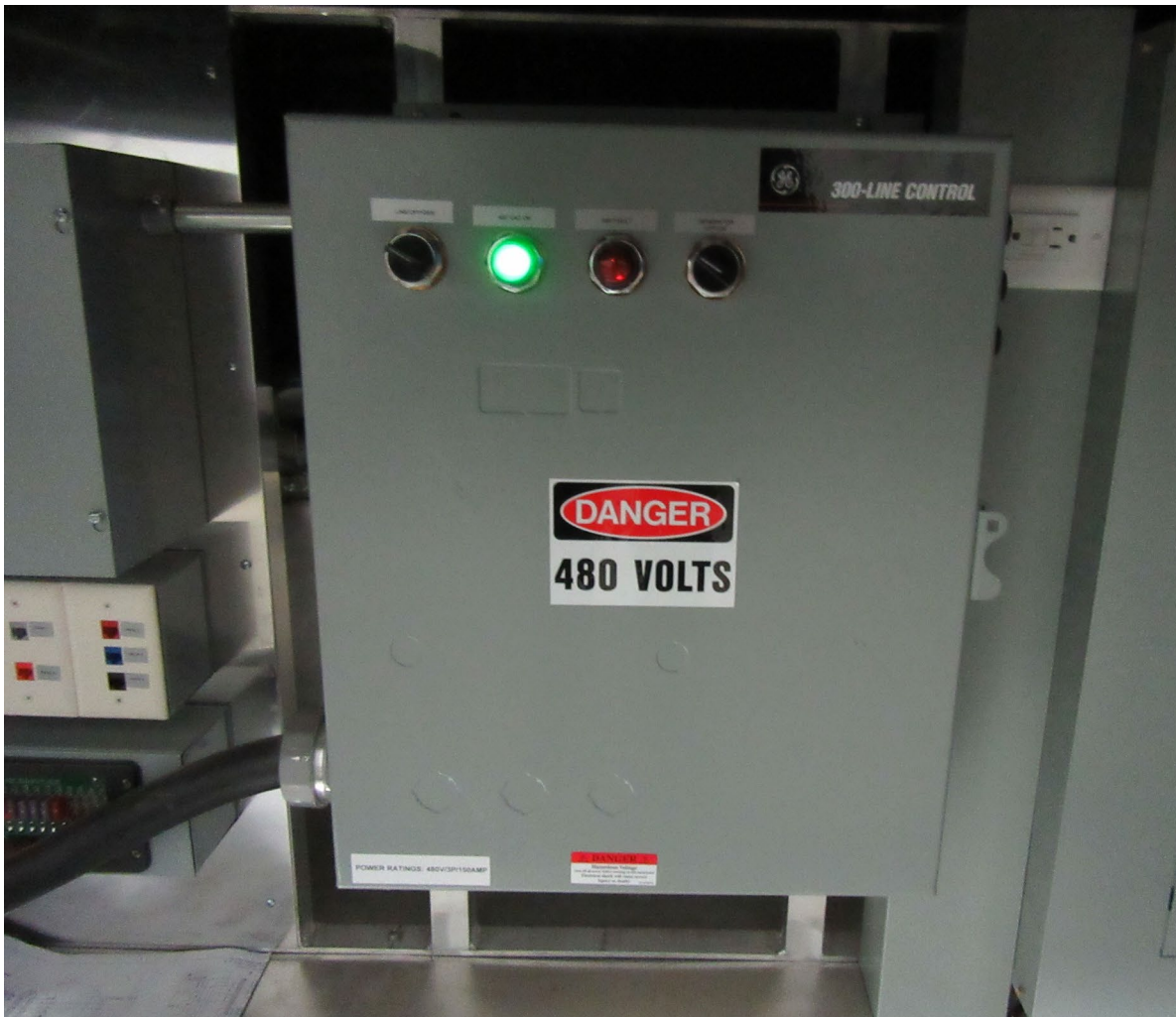
Figure 27: 480V AC Line Control Box
