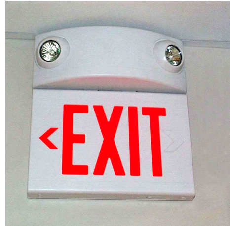
Figure 44: Emergency Dual Beam Lighting
