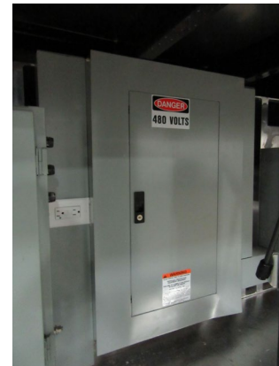
Figure 29: 480V AC Electrical Panel (Lower Compartment)
