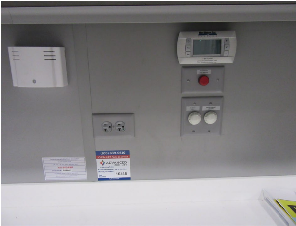
Controls at the Operators Console
