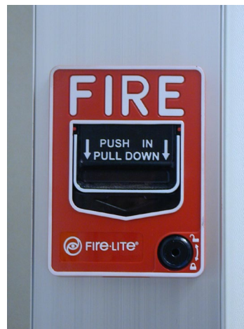
Figure 19: Fire Alarm Pull Station
