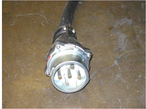
Figure 30: Shore Power Connection
