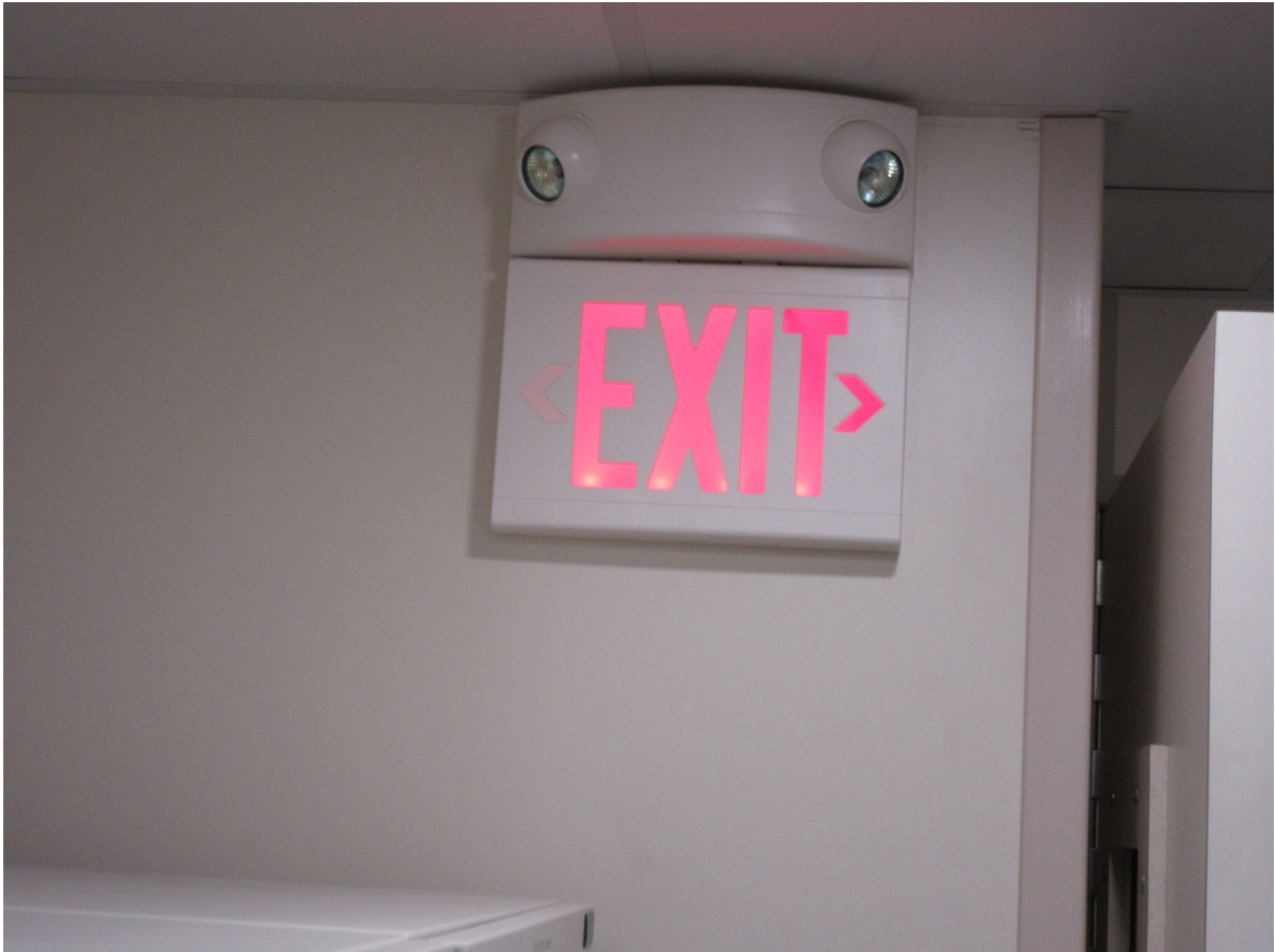
Figure 15: Control Room Emergency Lighting
