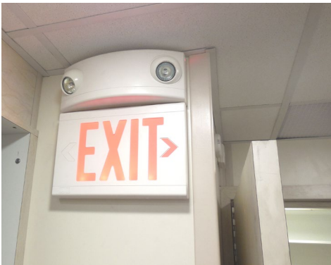
Control Room Emergency Light
