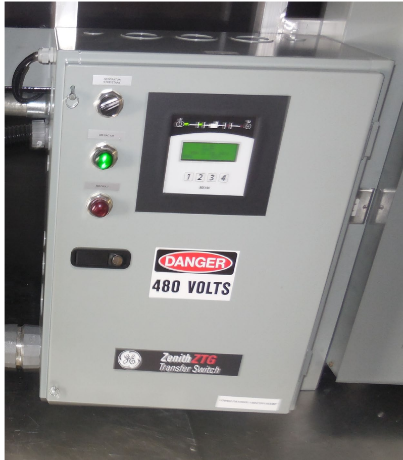
Figure 27: 480V AC ATS and Phase Power Monitor
