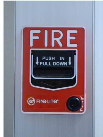
Figure 18: Fire Alarm Pull Station
