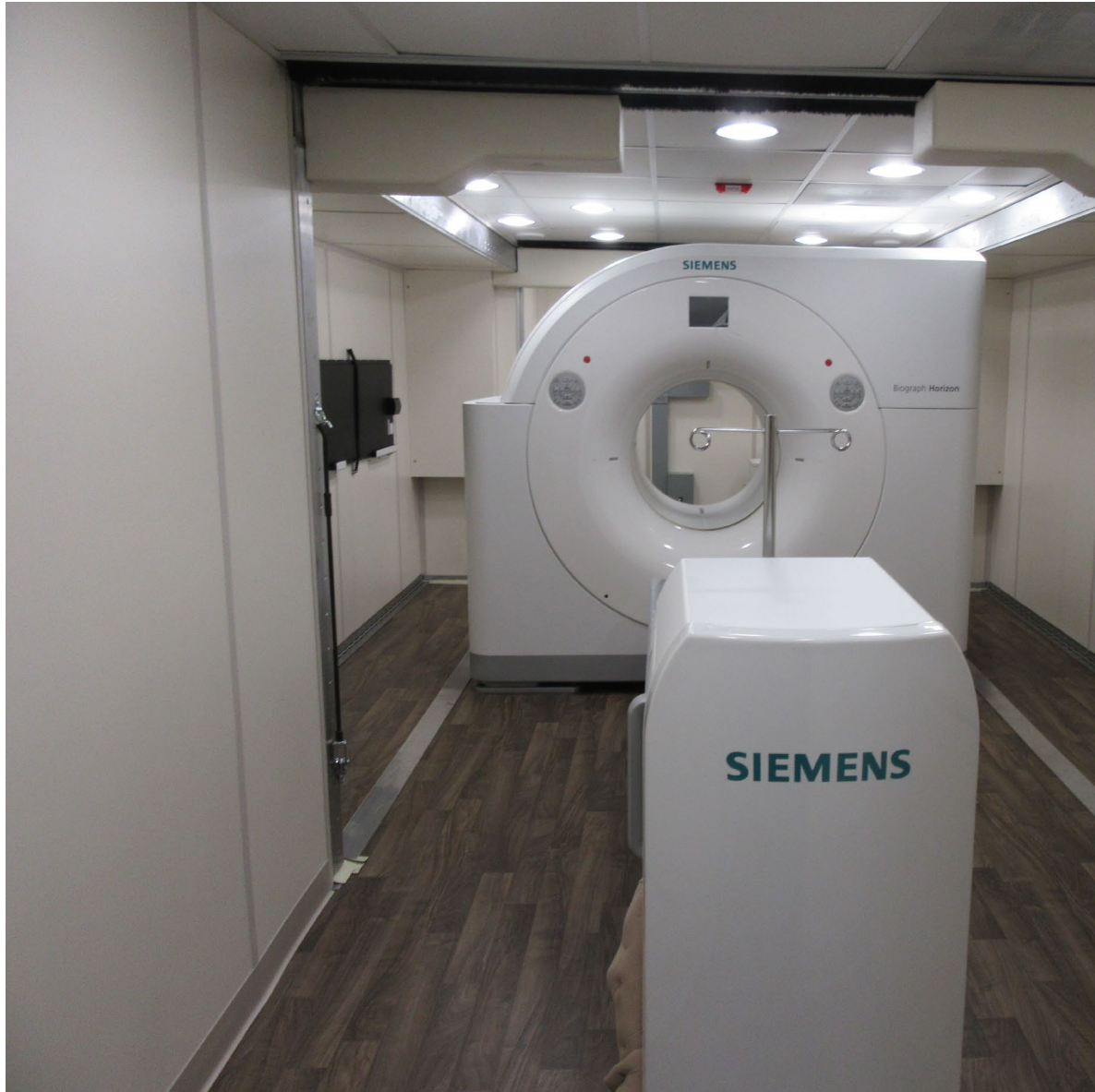
Figure 43: Gantry Room Overall Lighting
