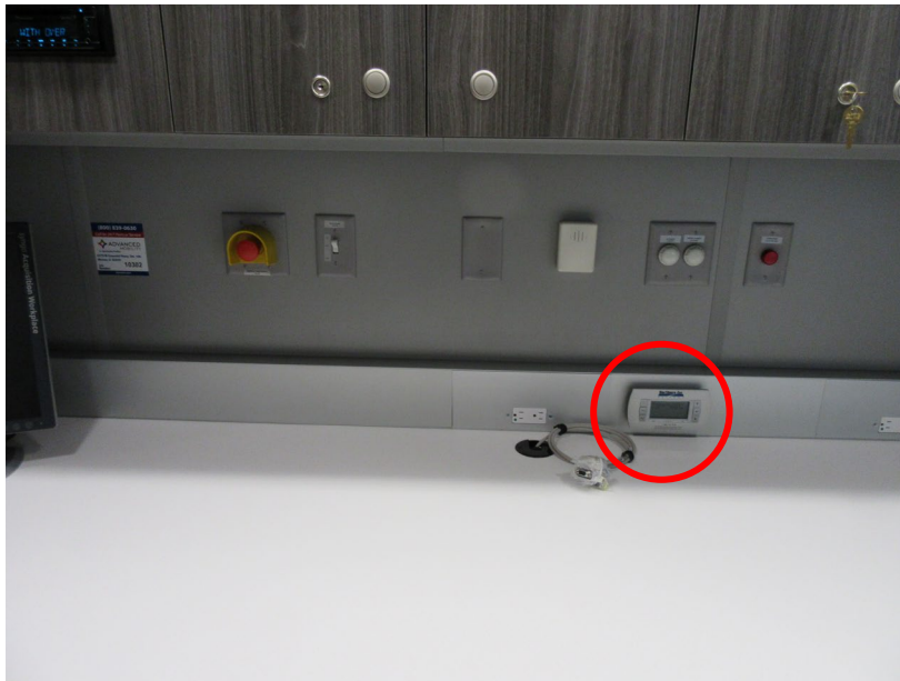
Remote Digital Displays for HVAC System in the Control Room to controls the Scan Room and the Control Room/Dispensing Lab
