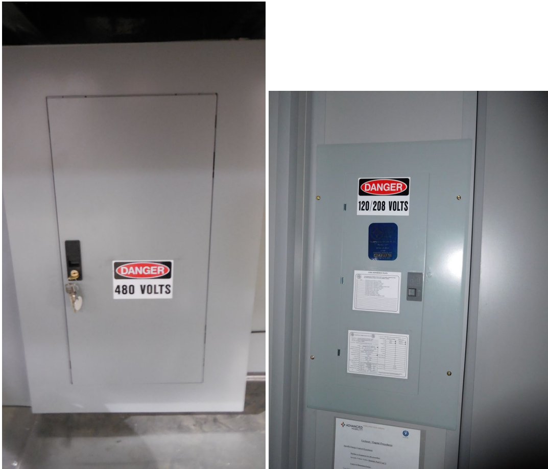
Figure 26: 480V and 120/208V AC Electrical Panels
