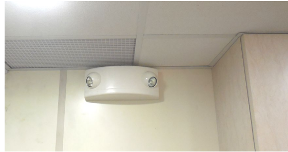
Gantry Room Emergency Light
