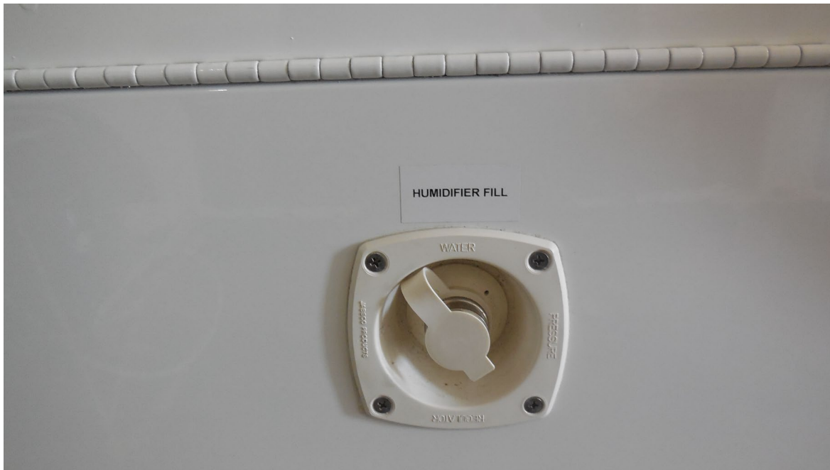
Figure 25: Humidifier Tank Fill
