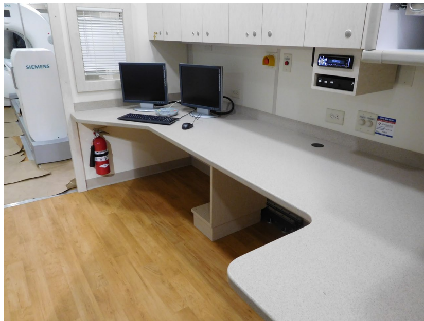
Scan Room and Control Room Light controls, and Humidifier low water level indicator lights.
