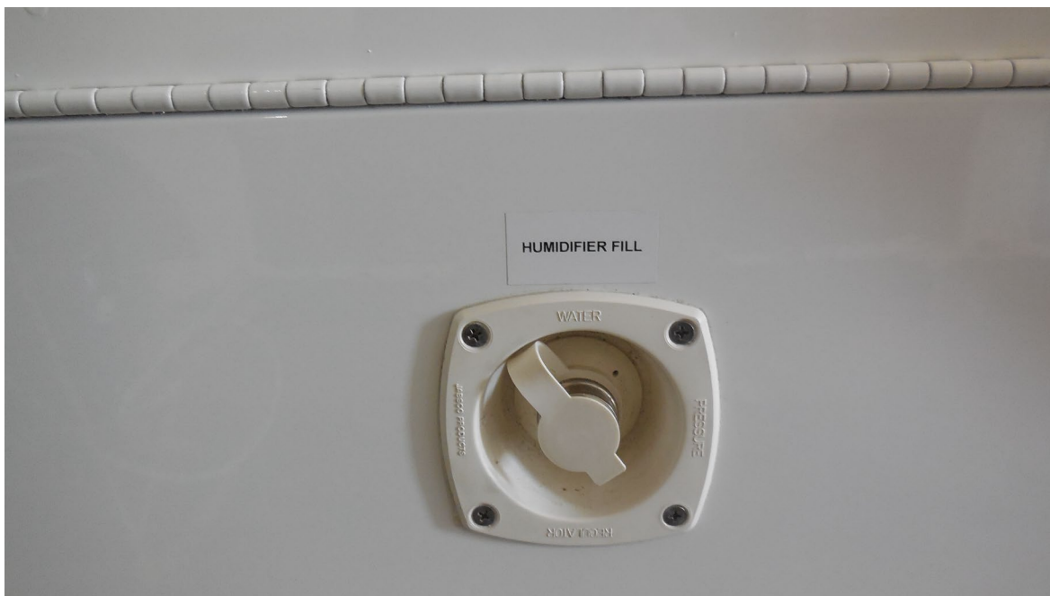
Figure 25: Humidifier Tank Fill
