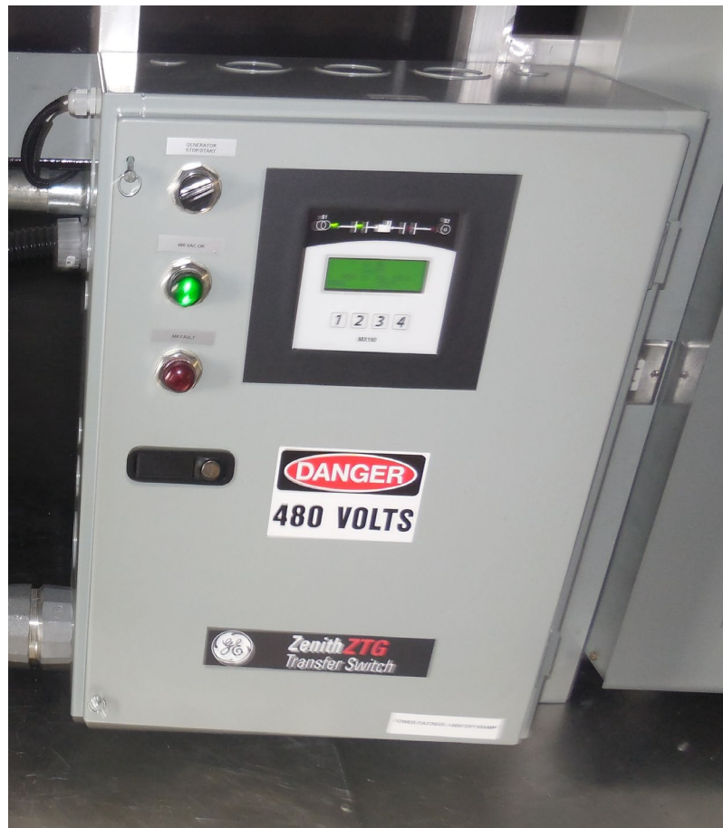
Figure 27: 480V AC ATS and Phase Power Monitor
