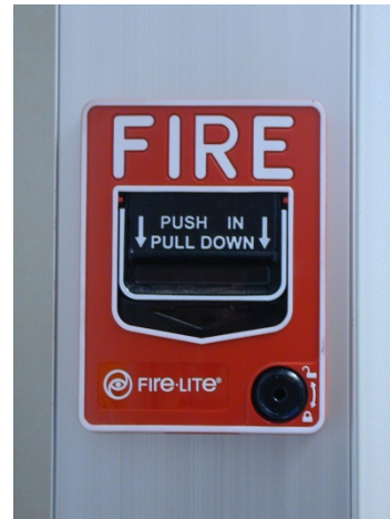
Figure 18: Fire Alarm Pull Station
