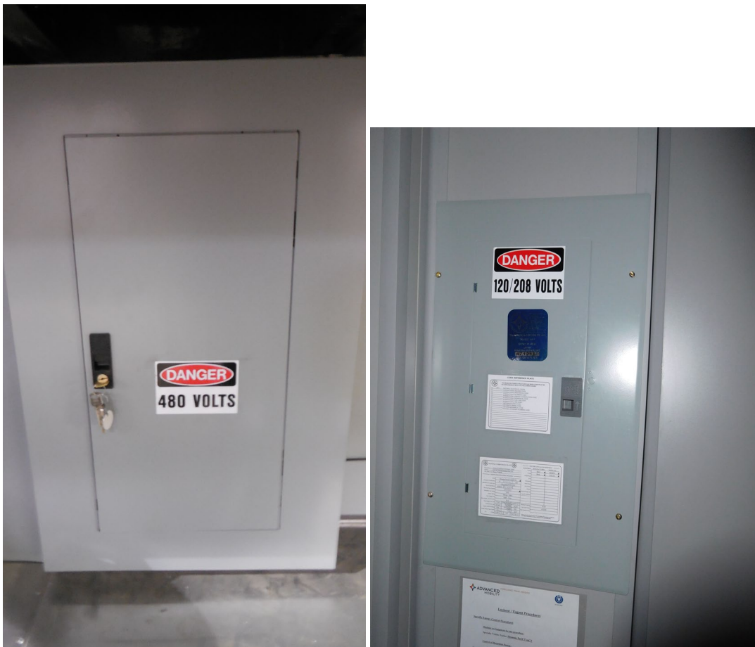
Figure 26: 480V and 120/208V AC Electrical Panels
