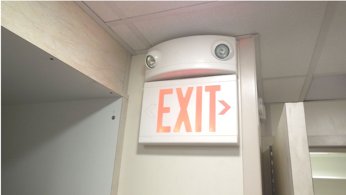
Figure 15: Control Room Emergency Lighting
