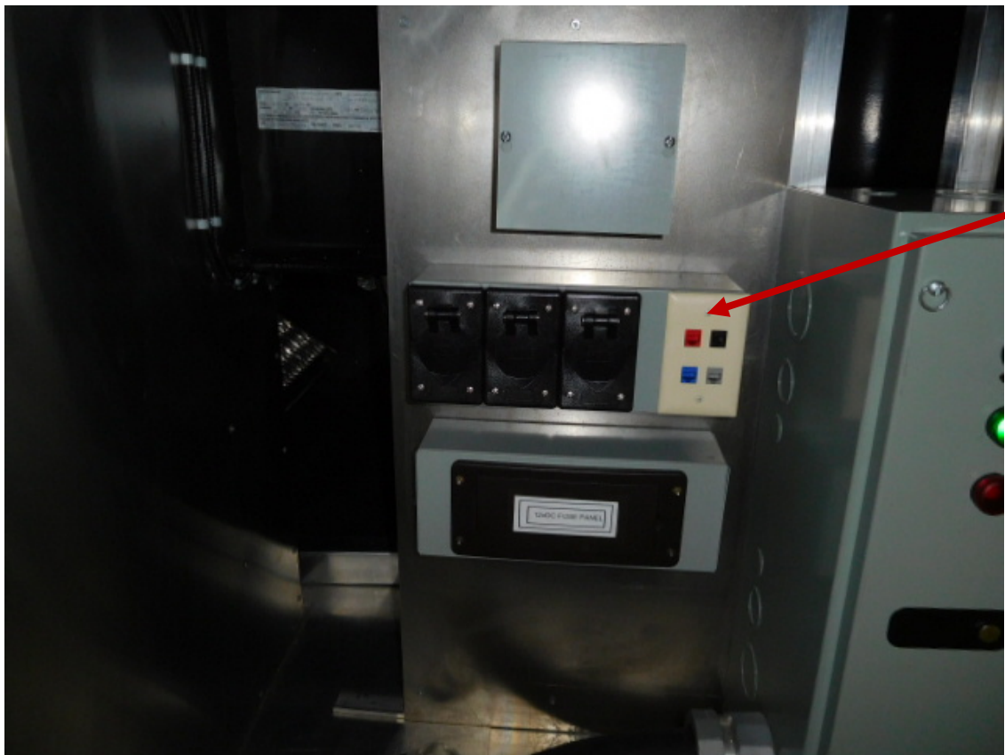
Figure 11: Phone & Data Line Connections
