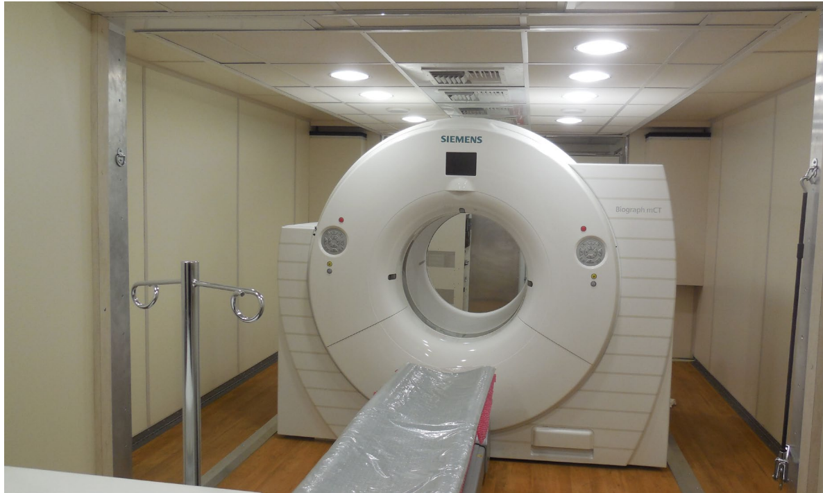
Figure 43: Gantry Room Overall Lighting
