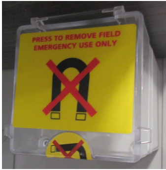
Guarded Magnet Quench Button, Scan Room
