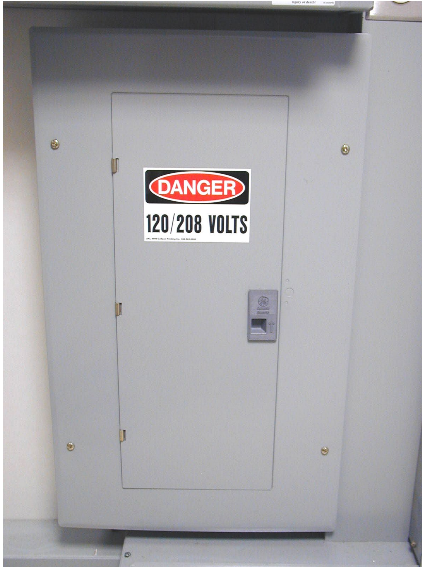
Figure 35: 120/208V AC Electrical Panel
