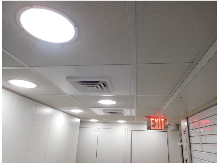
Figure 60: Control Room Lighting
