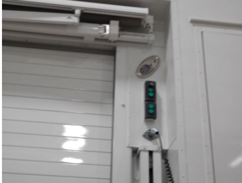
Right side LED Lighting
