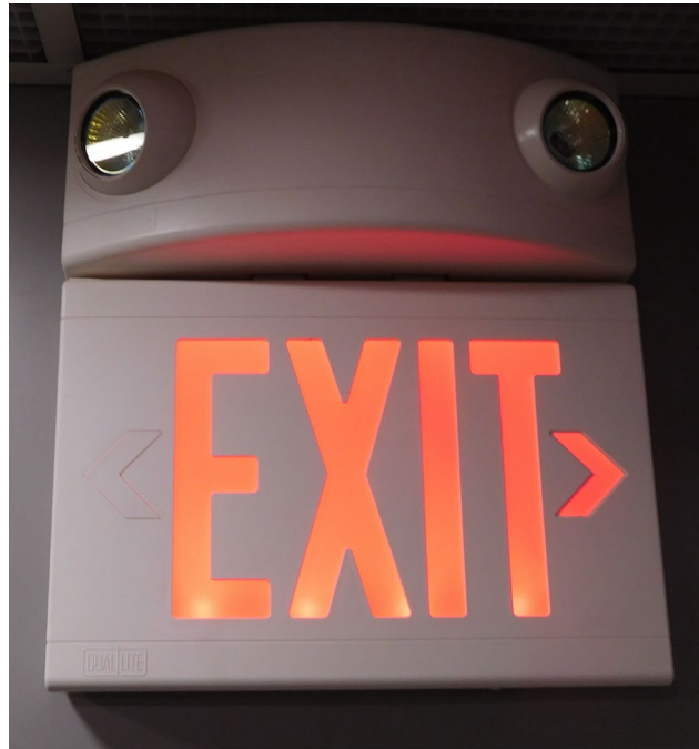
Figure 54: Emergency Dual Beam Lighting
