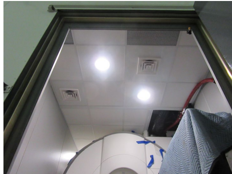
Magnet Room Lighting
