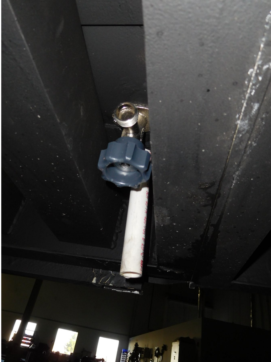
Figure 21: Fresh Water and Wastewater Connections
