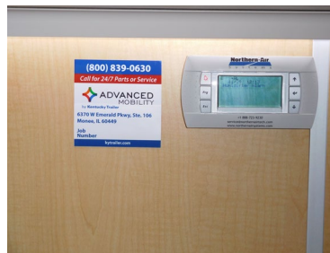
HVAC Monitor & Alarm
