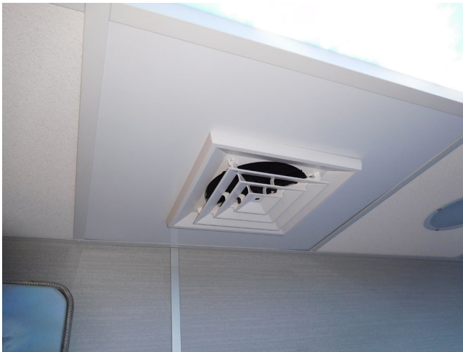
HVAC Vents Discharge
