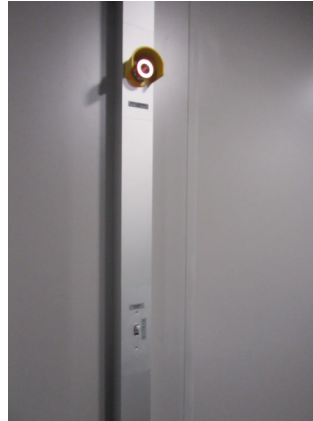
Emergency Off Button, Magnet Room
