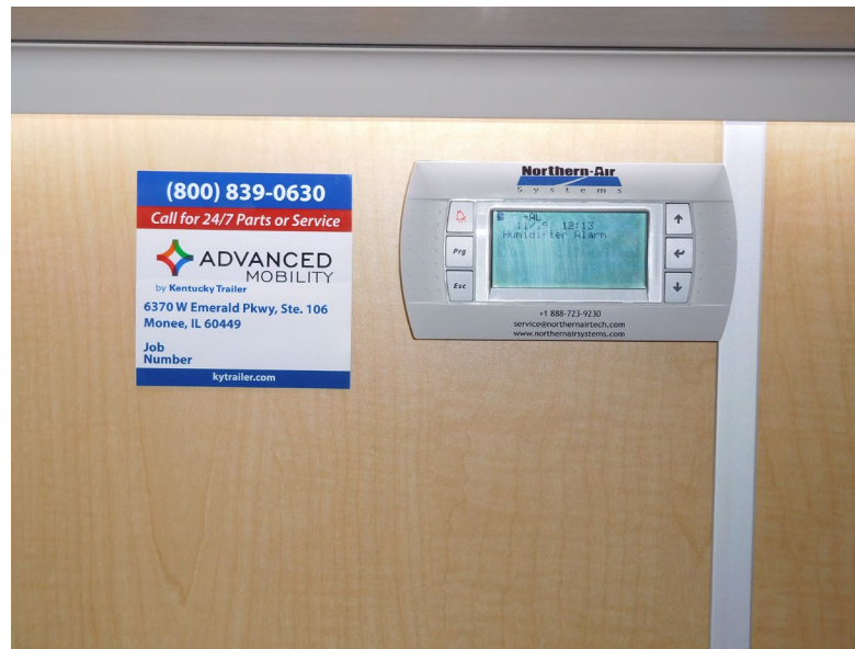
Figure 44: HVAC Monitor and Alarm Panel
