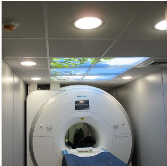
Figure 61: Scan Room Lighting
