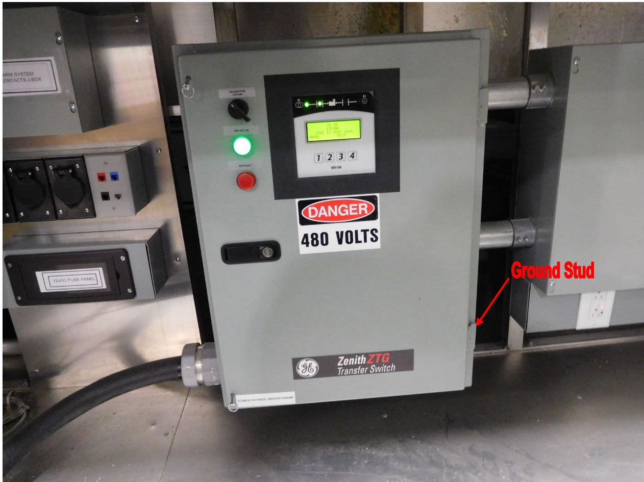
Figure 40: Power Supply Control Panel Ground Connection
