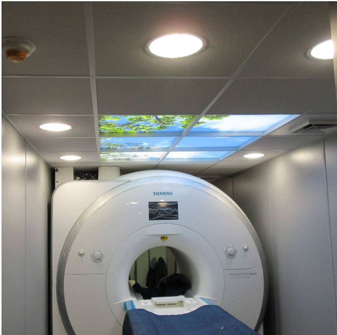
Figure 18: Scan Room Overall
