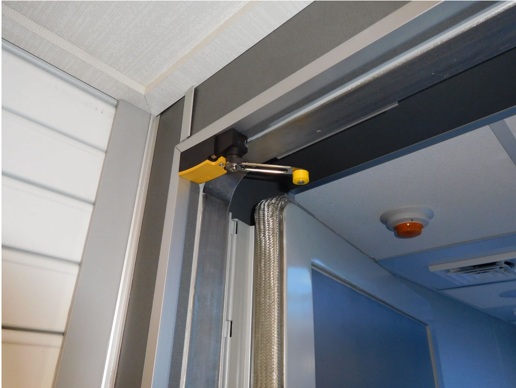
Close up of RF door trim
