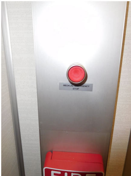
Emergency Off button, Control Room, next to Entry Door
