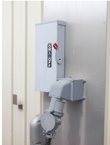
Figure 38: Shore Power Connection
