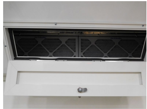
HVAC Filter Access
