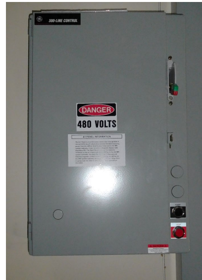
A1 Start/Stop in Equipment Room
