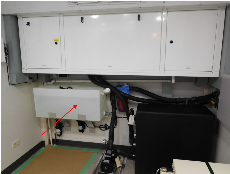
Figure 45: Humidifier Water Tank
