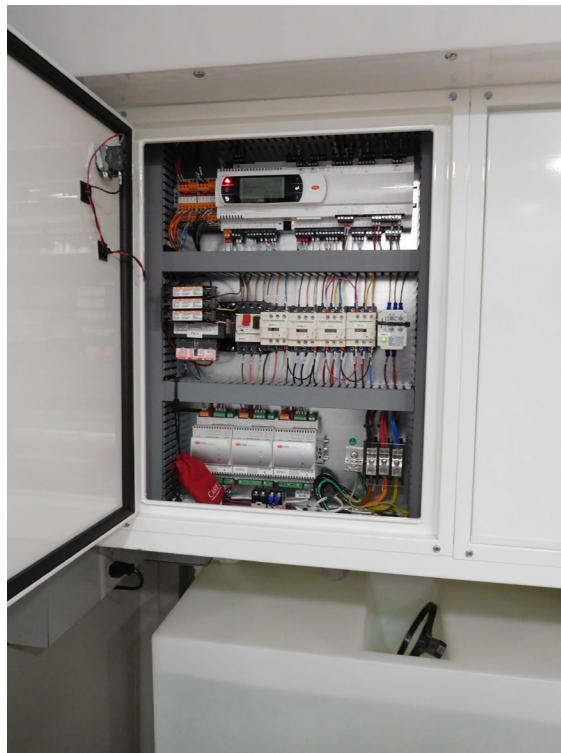
Figure 43: A/C / Chiller Control Panel
