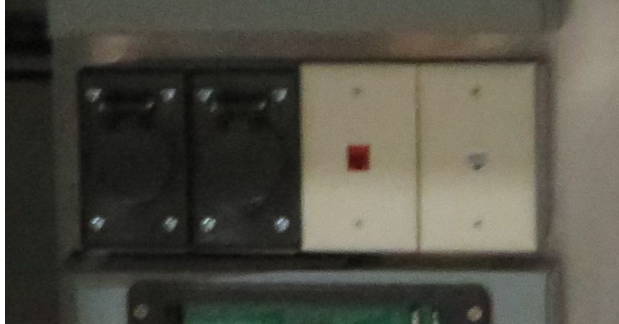
Figure 17: Phone & Data Line Connections
