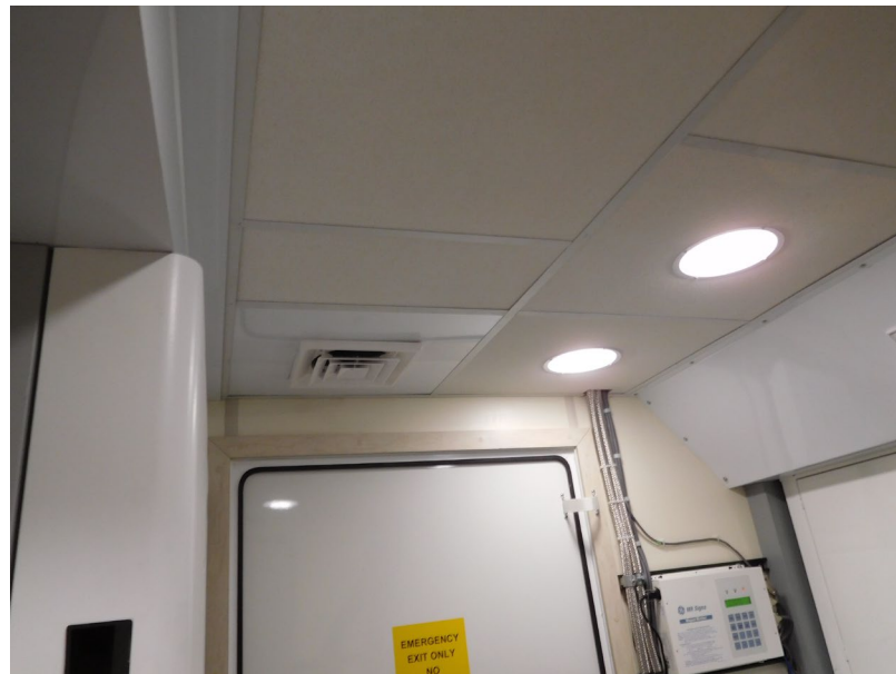
Figure 589: Equipment Room Lighting
