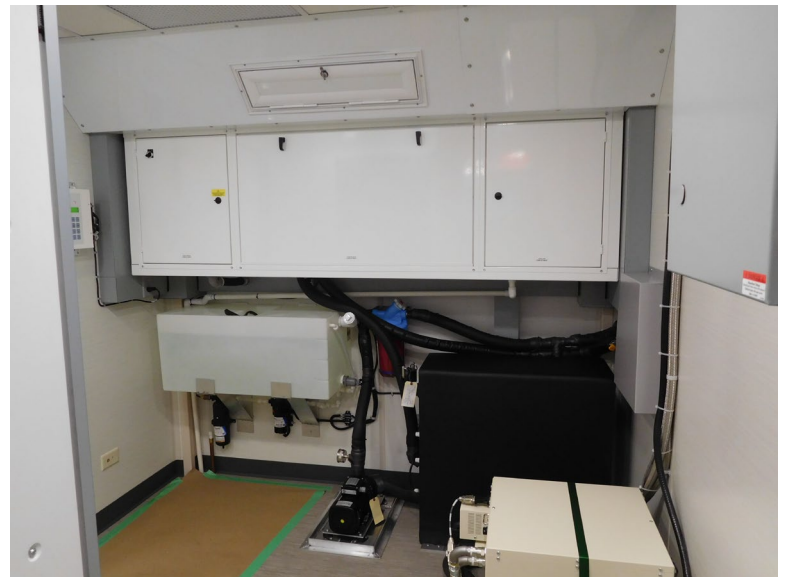
Figure 8: Equipment Room Overall
