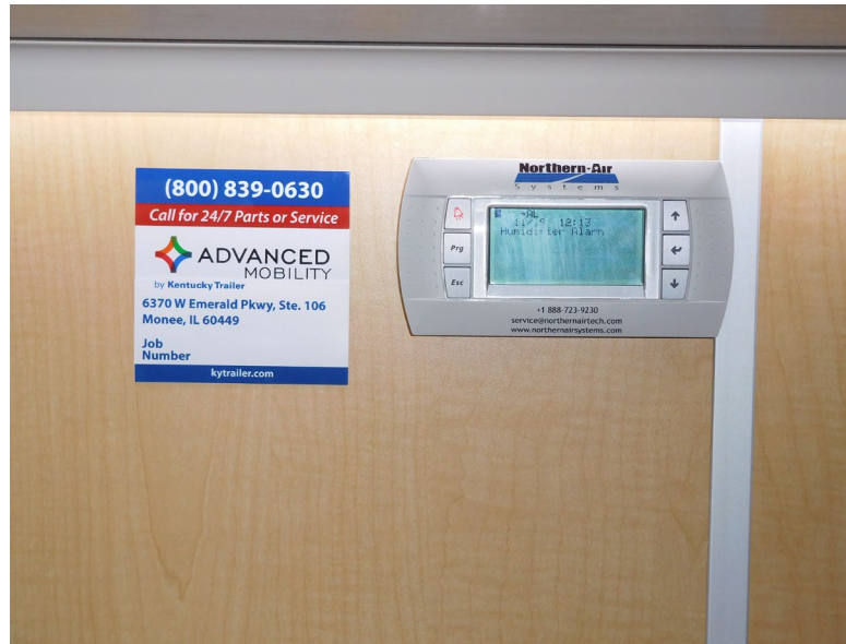
Figure 44: HVAC Monitor and Alarm Panel
