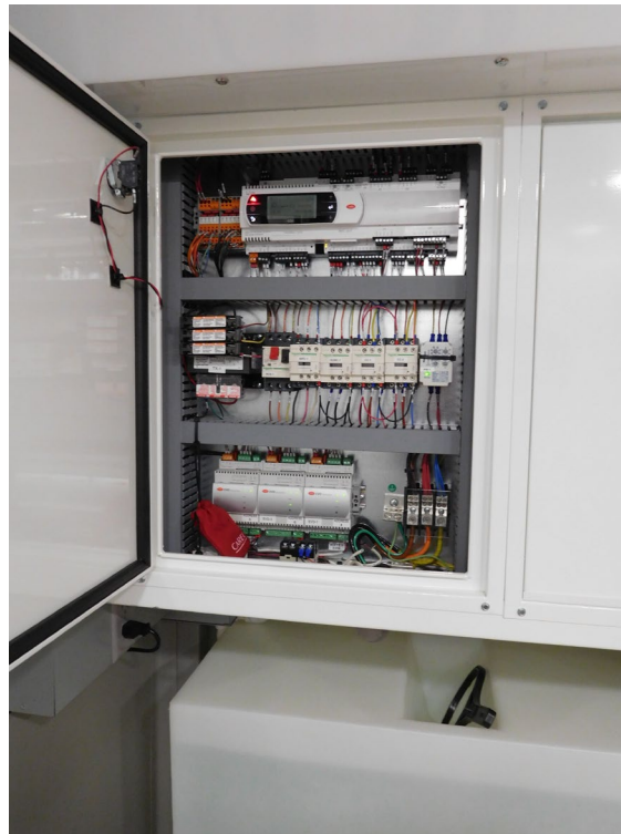
Figure 43: A/C / Chiller Control Panel
