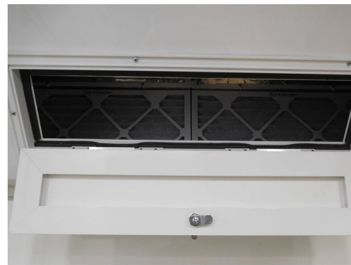
HVAC Filter Access
