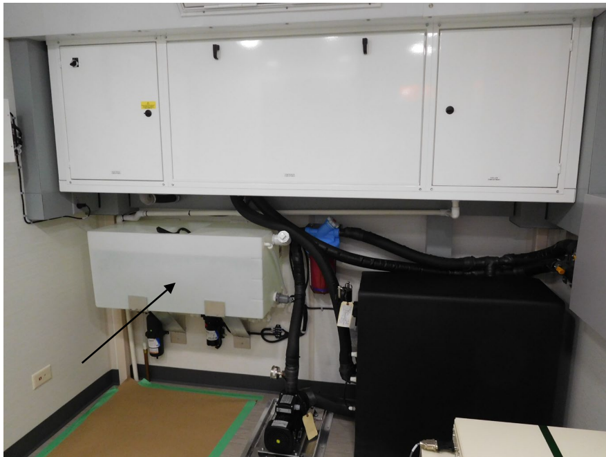
Figure 45: Humidifier Water Tank
