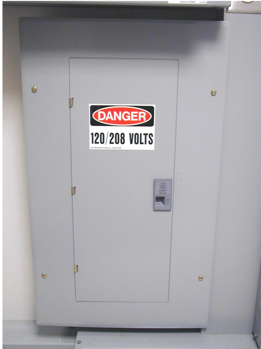
Figure 35: 120/208V AC Electrical Panel
