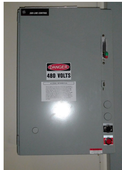
A1 Start/Stop in Equipment Room
