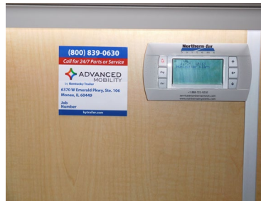
HVAC Monitor & Alarm
