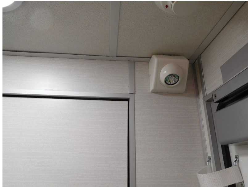
Figure 54: Emergency Dual Beam Lighting
