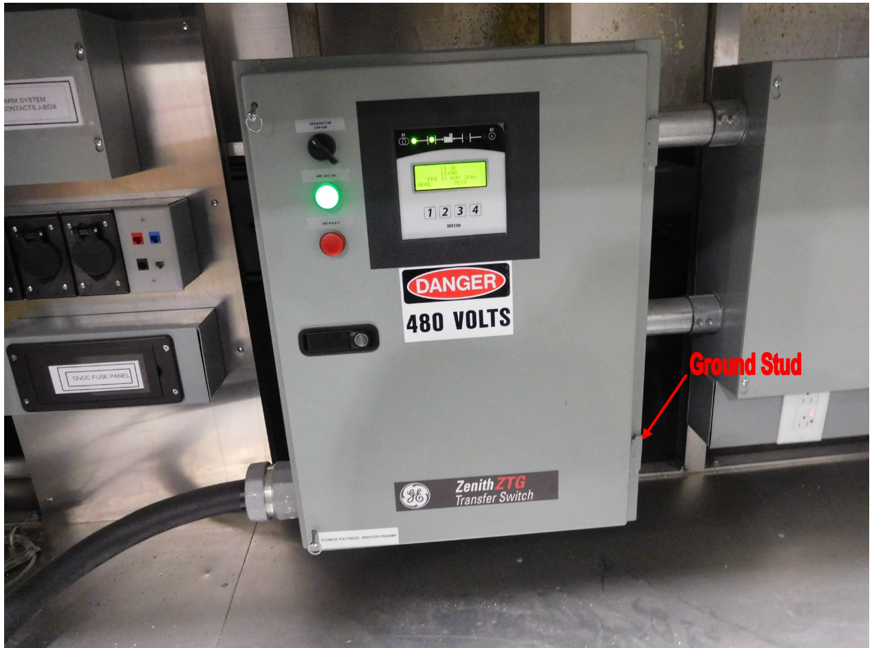
Figure 40: Power Supply Control Panel Ground Connection
