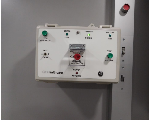
Guarded Magnet Quench Button, Scan Room
