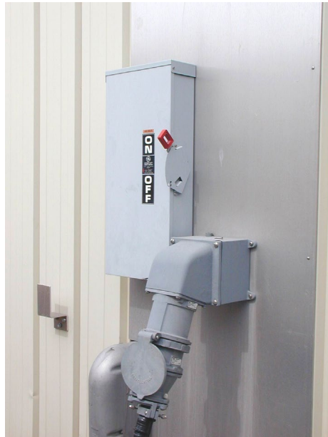
Figure 38: Shore Power Connection
