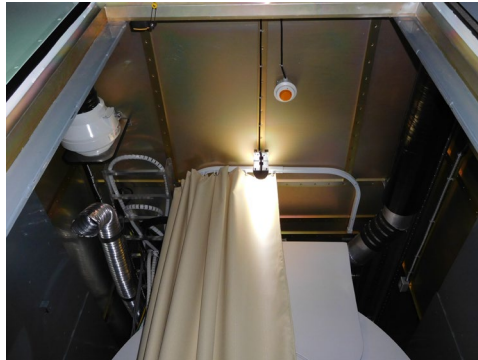
Magnet Room Lighting
