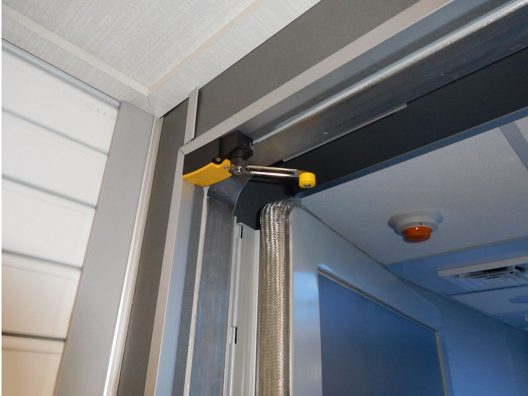
Close up of RF door trim
