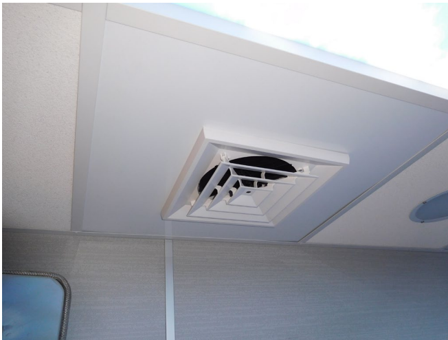
HVAC Vents Discharge
