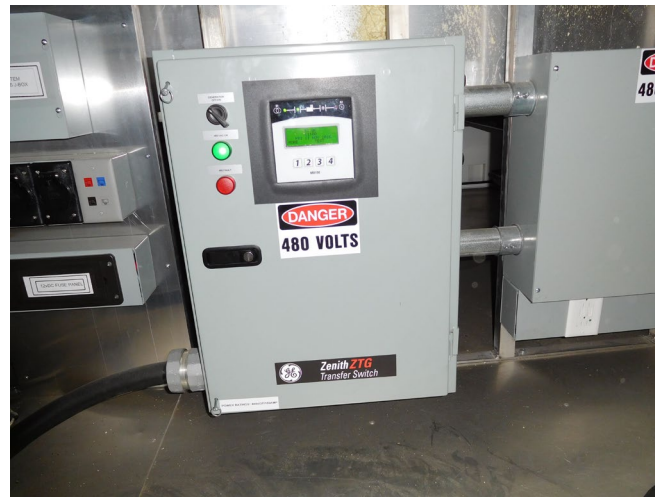
Figure 11: Power Supply Control Panel
