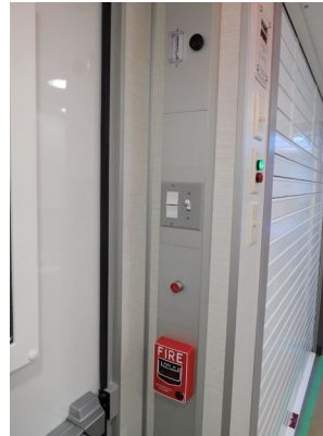
Control Room and Equipment Room Lighting and E-Stop Controls
