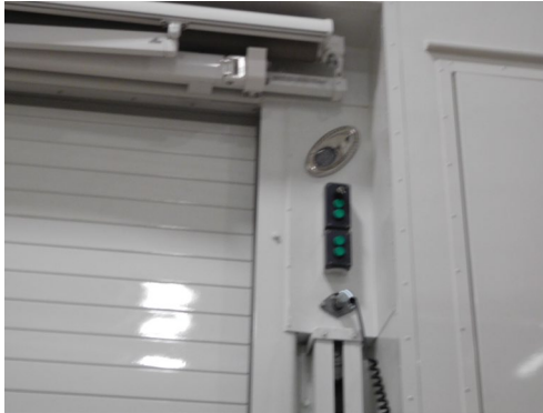
Right side LED Lighting
