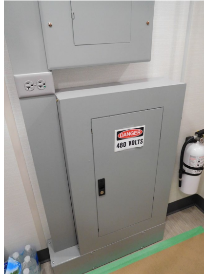
Figure 36: 480V AC Electrical Panel
