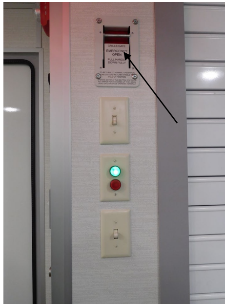
Figure 33: Roll Door Emergency Release
