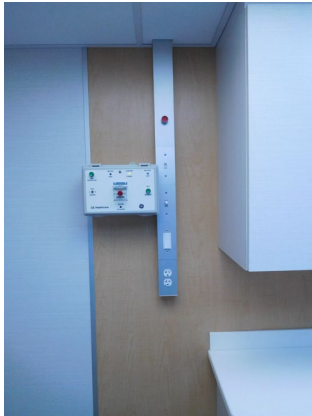
Scan Room and Magnet Room Lighting
