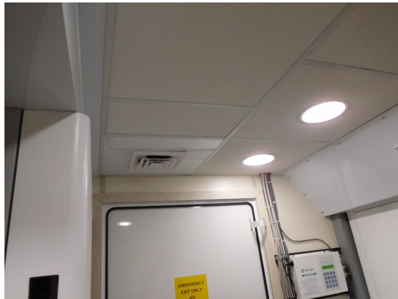
Figure 589: Equipment Room Lighting
