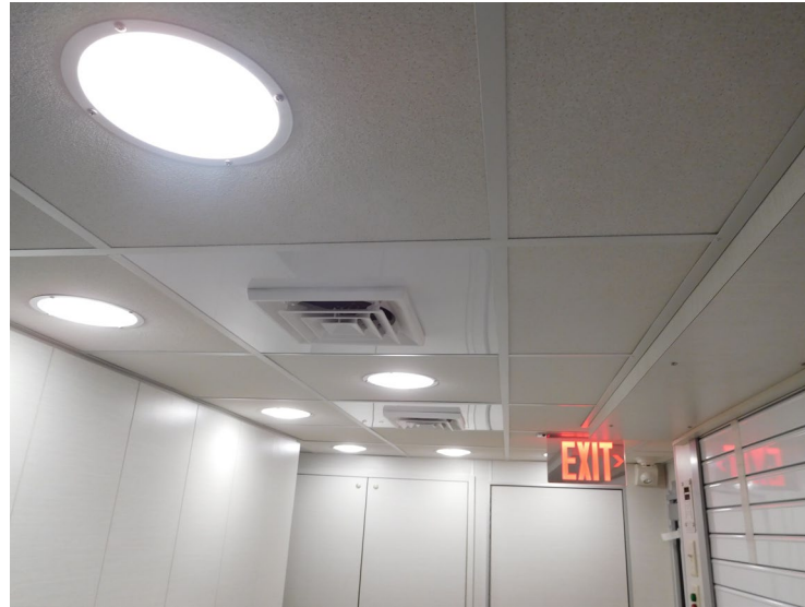
Figure 60: Control Room Lighting
