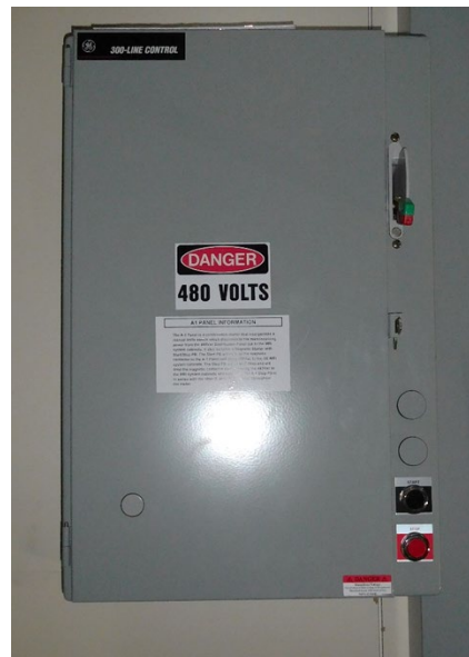
Figure 37: A1 Electrical Panel
