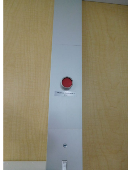
Emergency Off Button, Magnet Room
