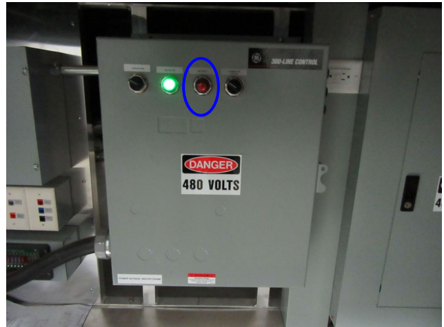
Figure 51: 480V AC Fault Indicator Light
