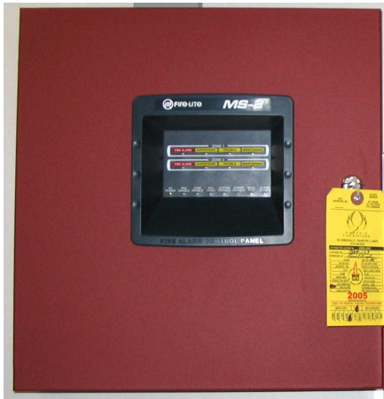
Figure 18: Fire Alarm Control Panel
