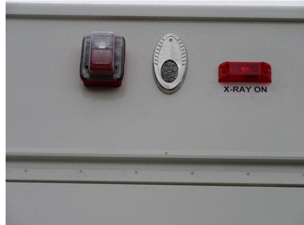
Figure 47: Staff Door Lighting
