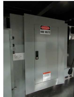
Figure 29: 480V AC Electrical Panel (Lower Compartment)
