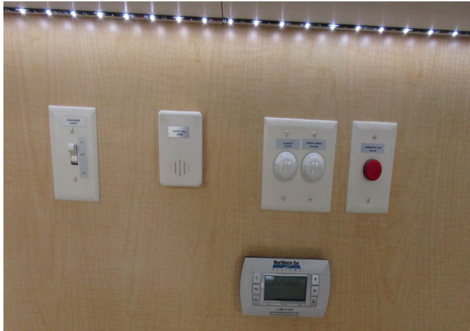
Controls at the Operators Console
