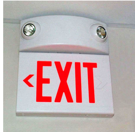
Figure 44: Emergency Dual Beam Lighting
