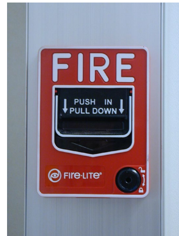
Figure 19: Fire Alarm Pull Station
