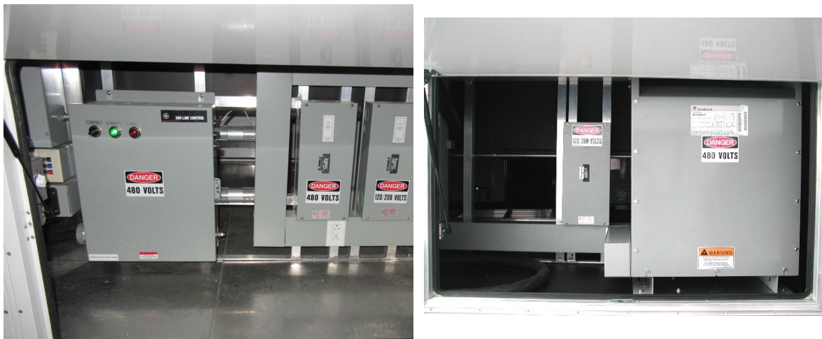
Figure 28: 480V AC Electrical Panel (underbody)
