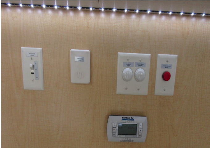
Controls at the Operators Console
