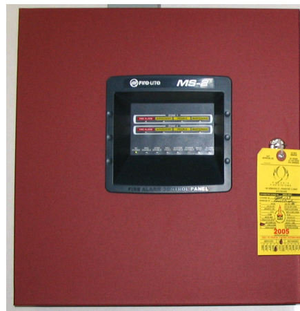
Figure 18: Fire Alarm Control Panel
