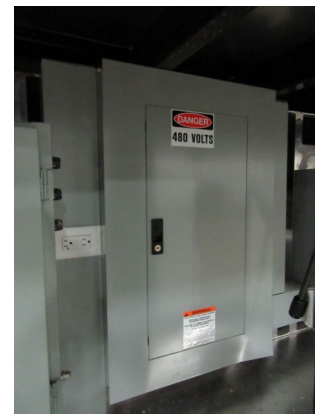
Figure 29: 480V AC Electrical Panel (Lower Compartment)
