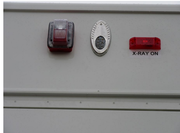
Figure 47: Staff Door Lighting
