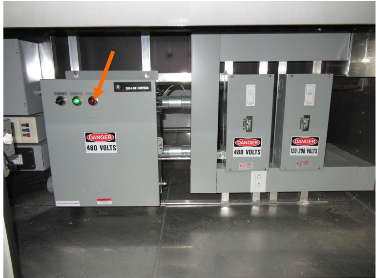
Figure 51: 480V AC Fault Indicator Light
