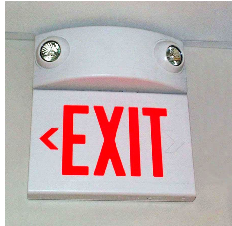
Figure 44: Emergency Dual Beam Lighting
