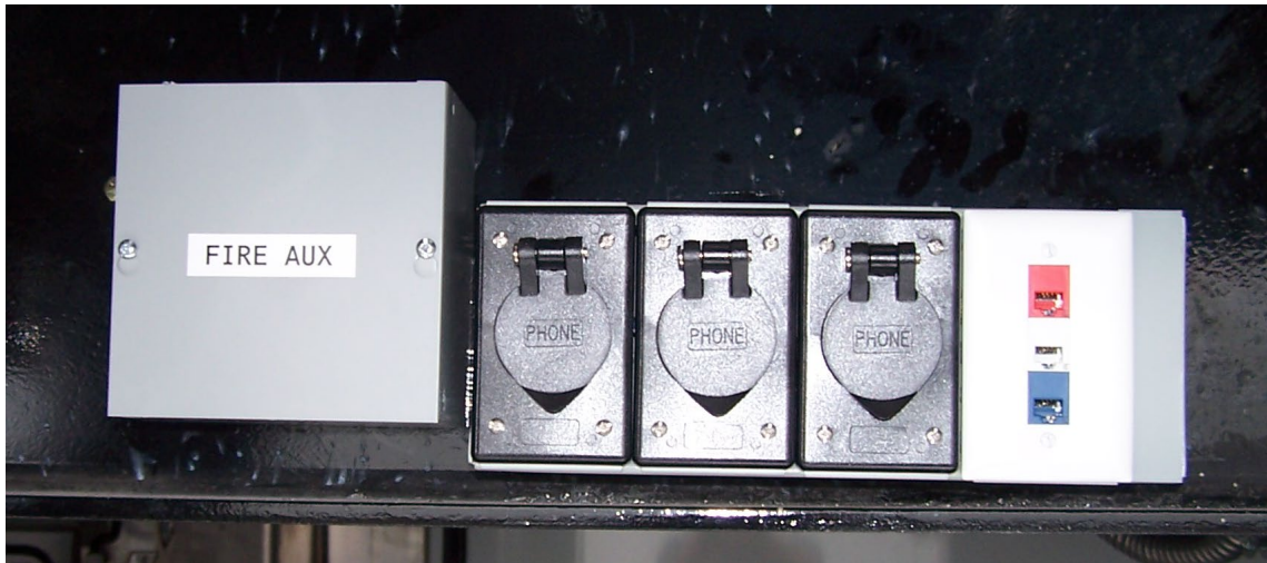
Figure 12: Phone & Data Line Connections
