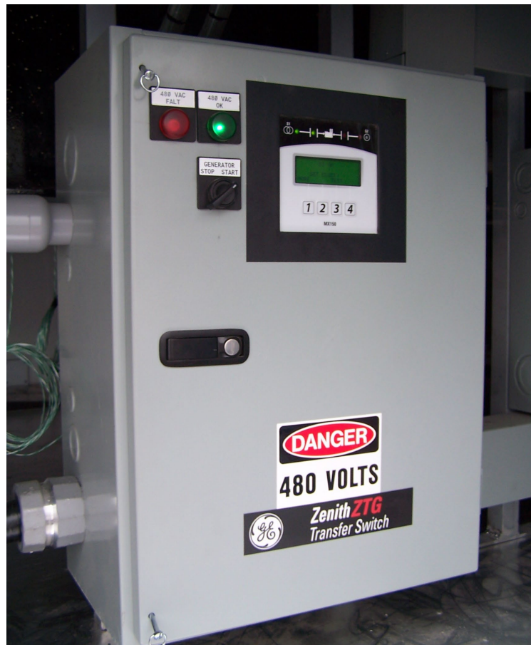
Figure 25: 480V AC ATS and Phase Power Monitor
