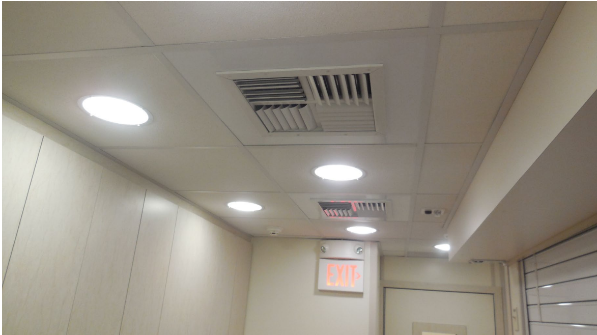
Figure 41: Control Room Overall Lighting
