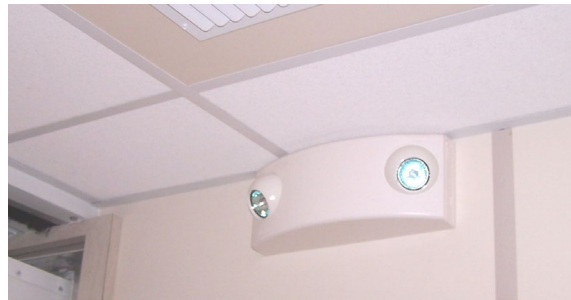
Gantry Room Emergency Light
