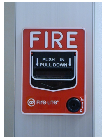
Figure 20: Fire Alarm Pull Station
