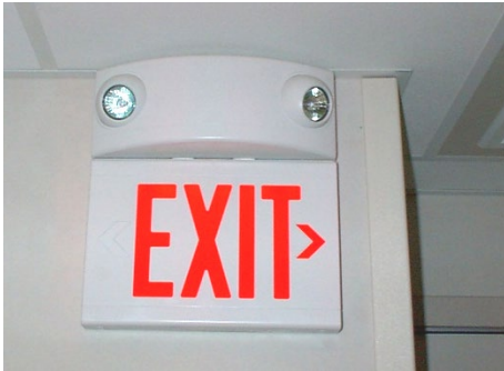
Control Room Emergency Light
