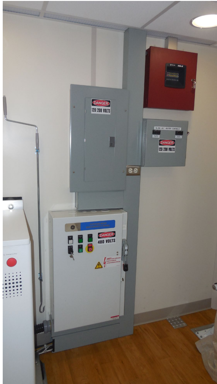
Figure 24: 120/208V AC Electrical Panels
