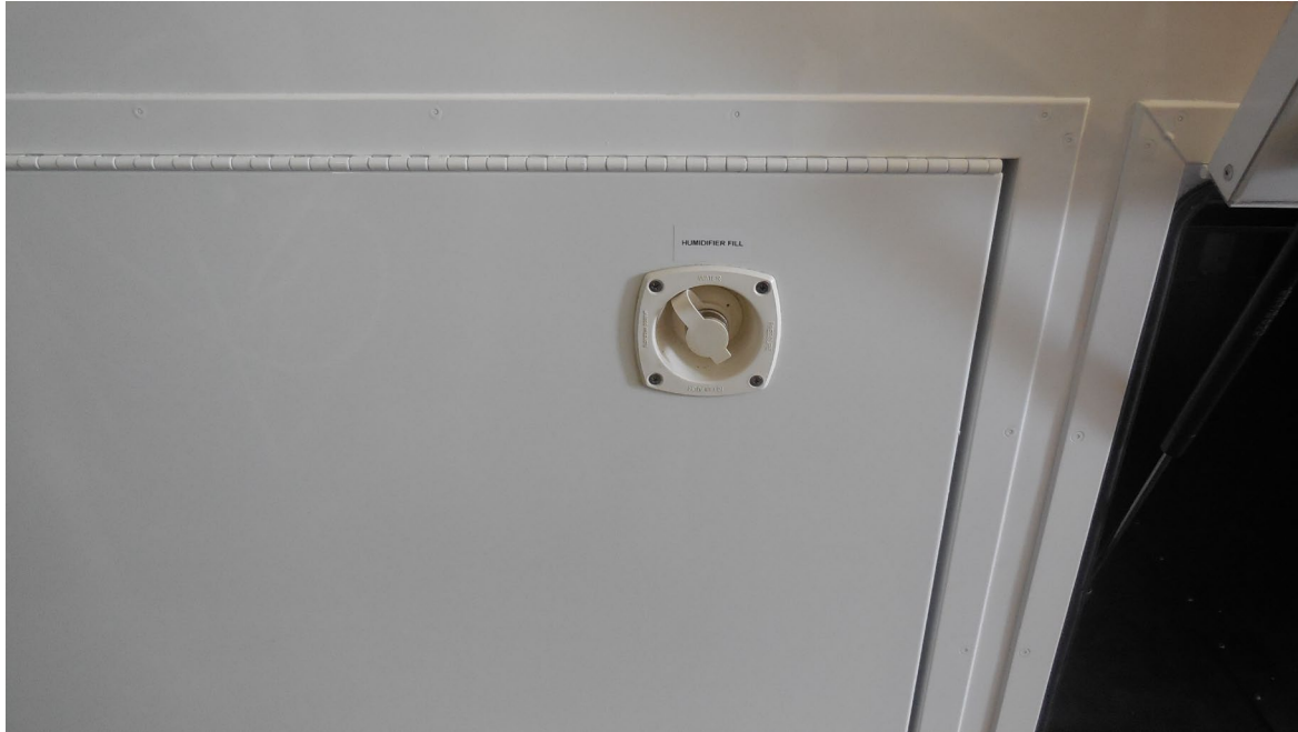
Figure 23: Humidifier Tank Fill
