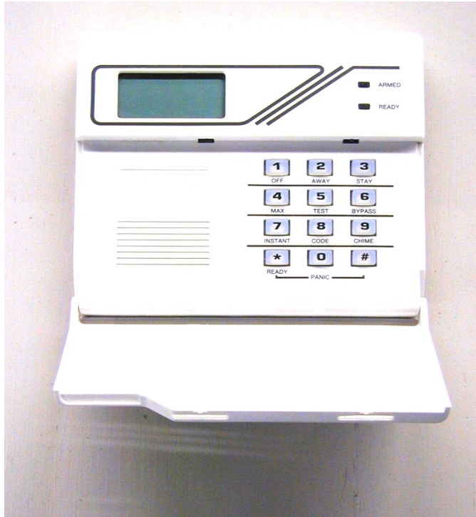
Figure 35: Intrusion Alarm Keypad
