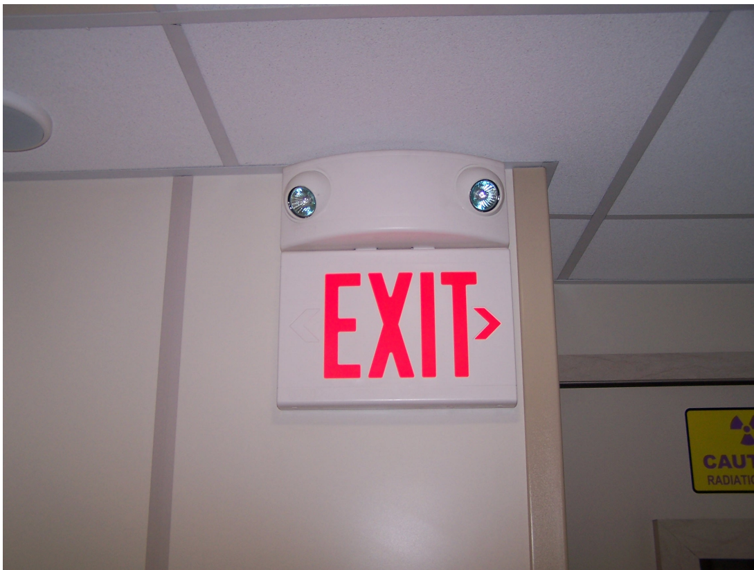
Figure 16: Control Room Emergency Lighting
