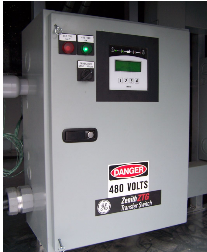
Figure 22: Automatic Transfer Switch and Phase Power Monitor
