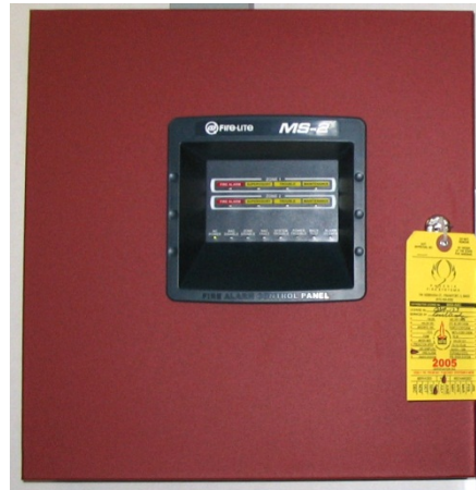
Figure 19: Fire Alarm Control Panel
