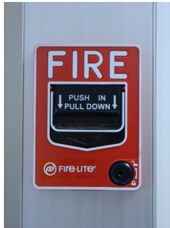
Figure 24: Fire Alarm Pull Station
