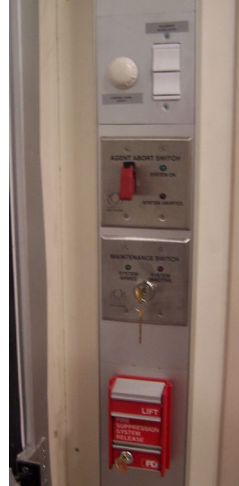
Control Room Lighting and E-Stop
