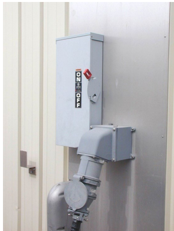
Figure 33: Shore Power Connection
