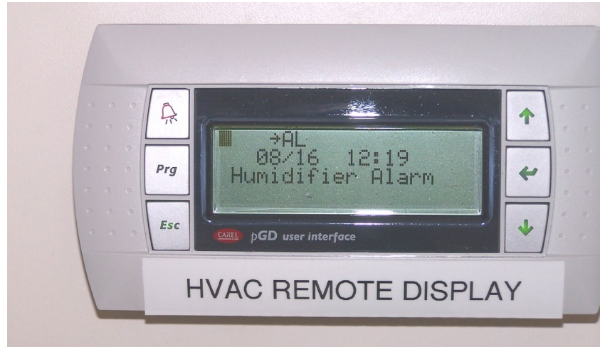
Figure 40: HVAC Remote Digital Display Panel
