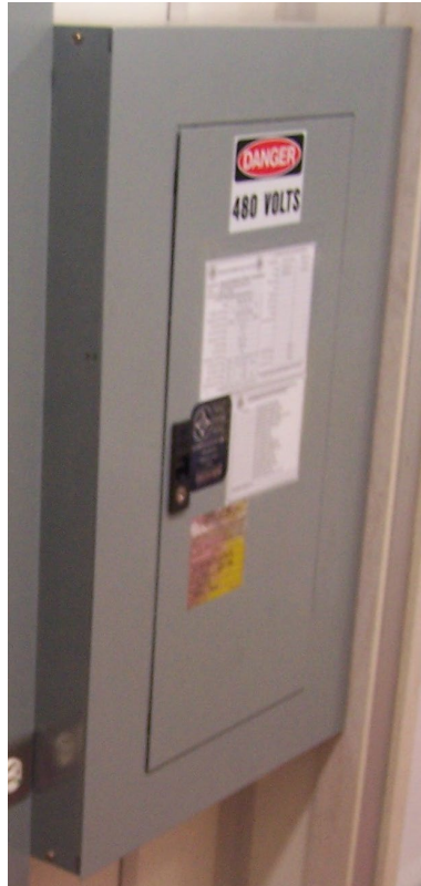
Figure 32: 480V AC Electrical Panel
