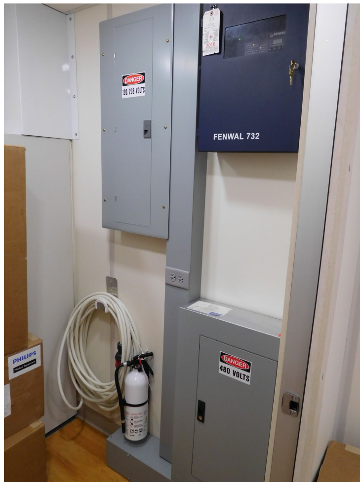
120/208V AC Distribution Panel
