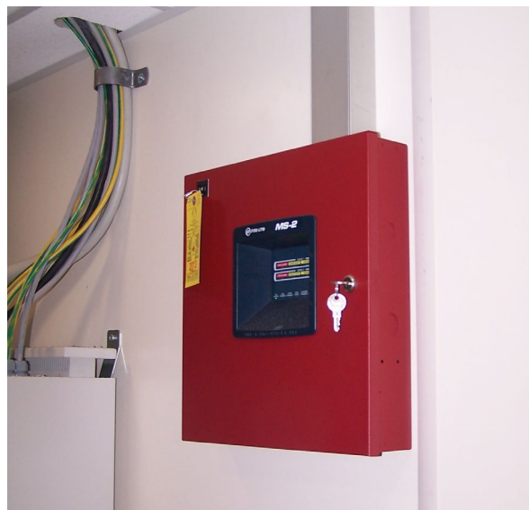
Figure 23: Fire Alarm Control Panel
