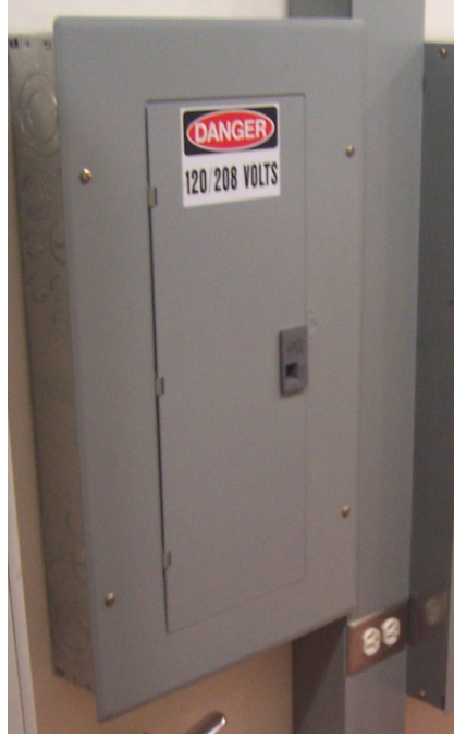
Figure 31: 120 / 208V AC Electrical Panel
