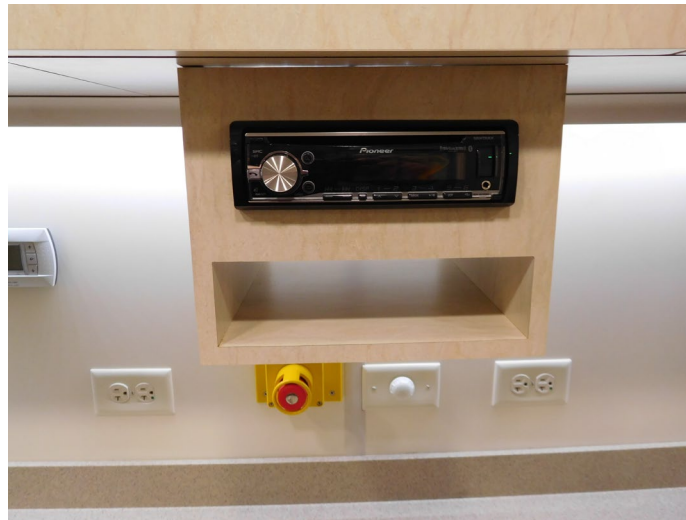
Figure 4: Control Room Overall
