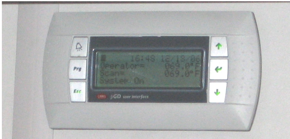
Air Conditioning Remote Status Annunciator & Alarm Panel
