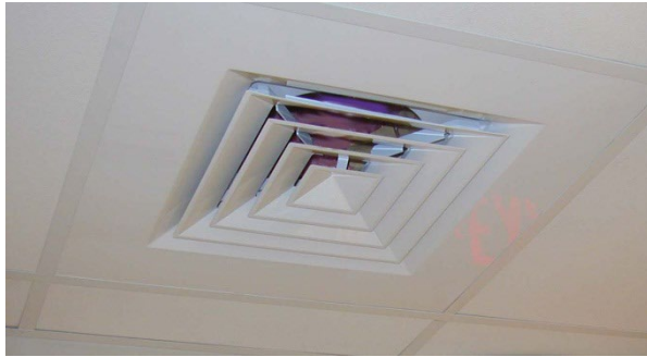
HVAC Vents Discharge
