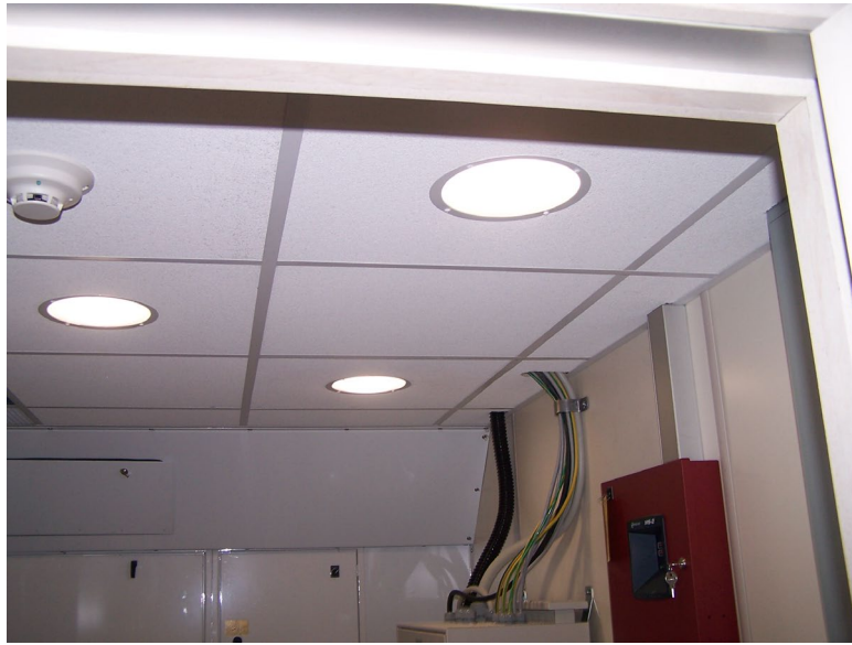
Figure 50: Equipment Room Lighting
