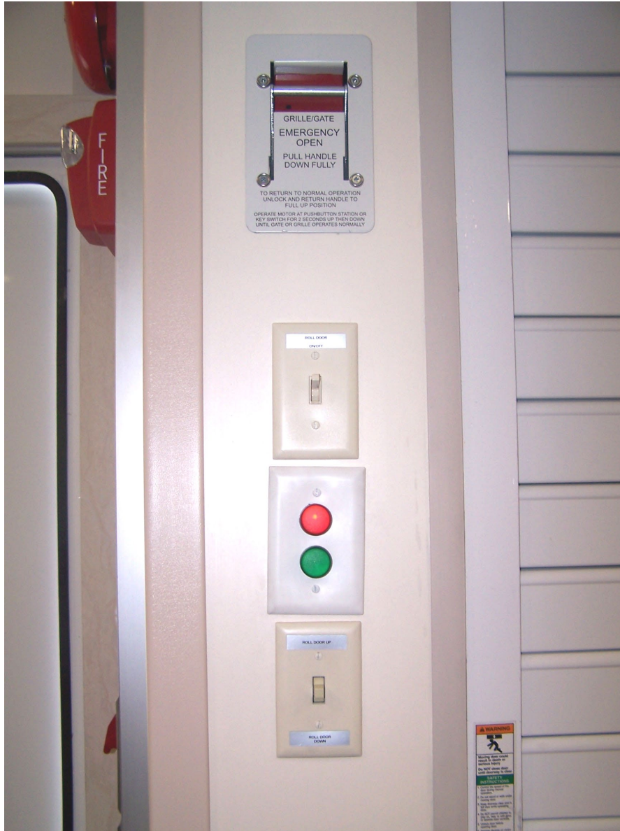
Figure 29: Roll Door Emergency Release
