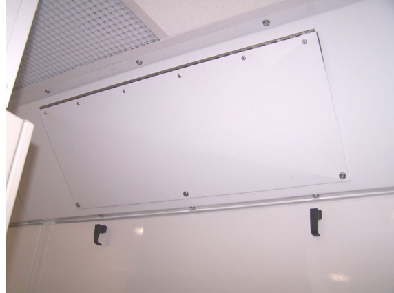
HVAC Filter Access
