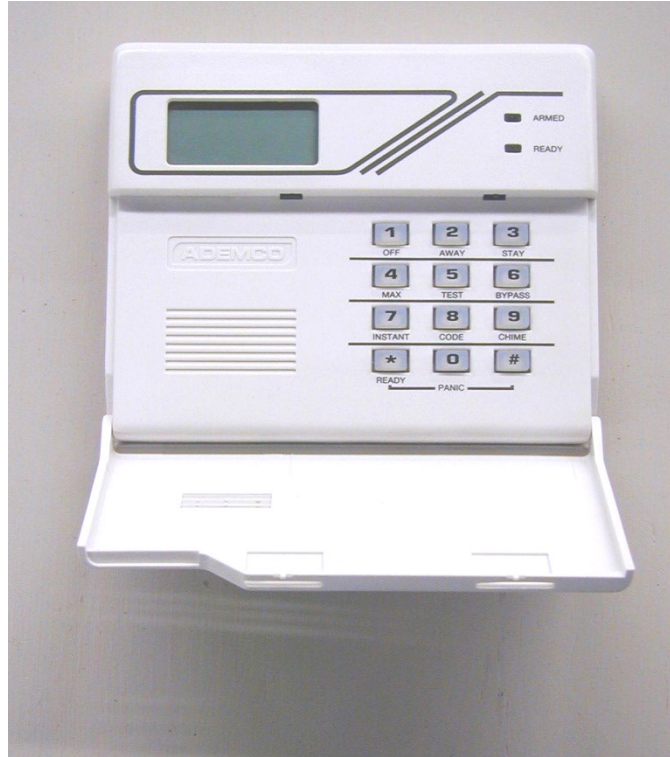
Figure 45: Intrusion Alarm Keypad
