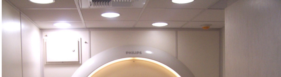
Figure 52: Scan Room Lighting
