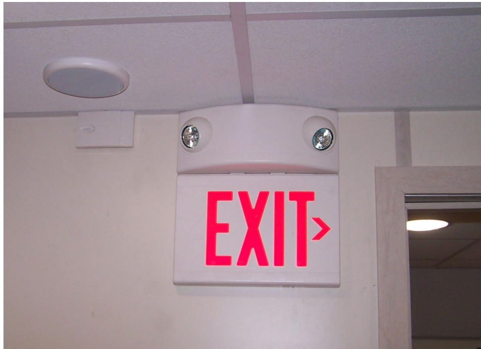
Figure 48: Emergency Dual Beam Lighting
