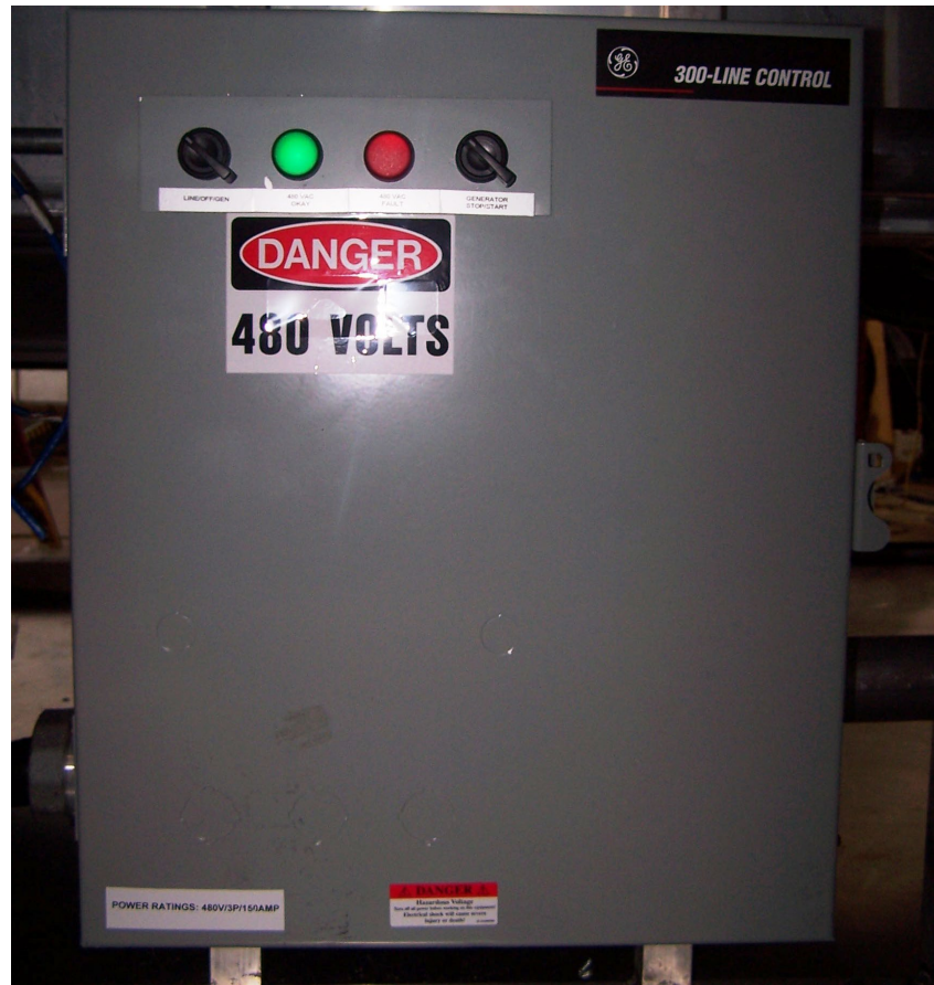
Figure 9: Power Supply Control Panel
