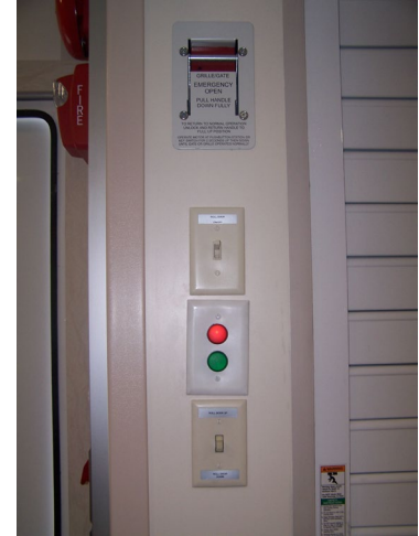
Roll Door Controls and Platform lift "UP" light
