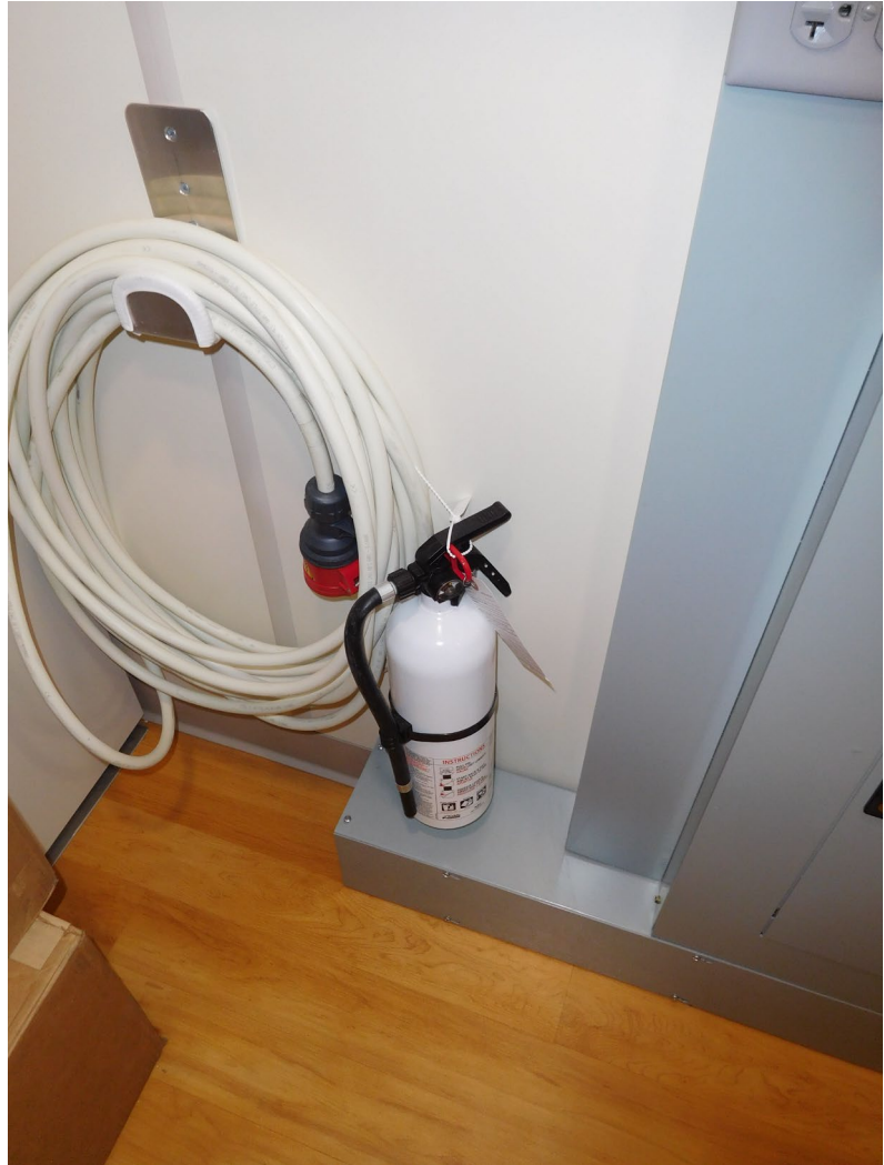
Figure 21: Fire Extinguisher (Typical)
