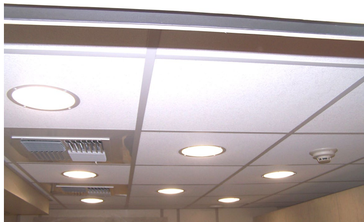
Figure 51: Control Room Lighting
