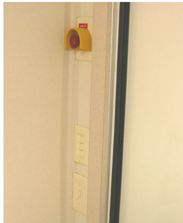
Control Room Lighting and E-Stop
