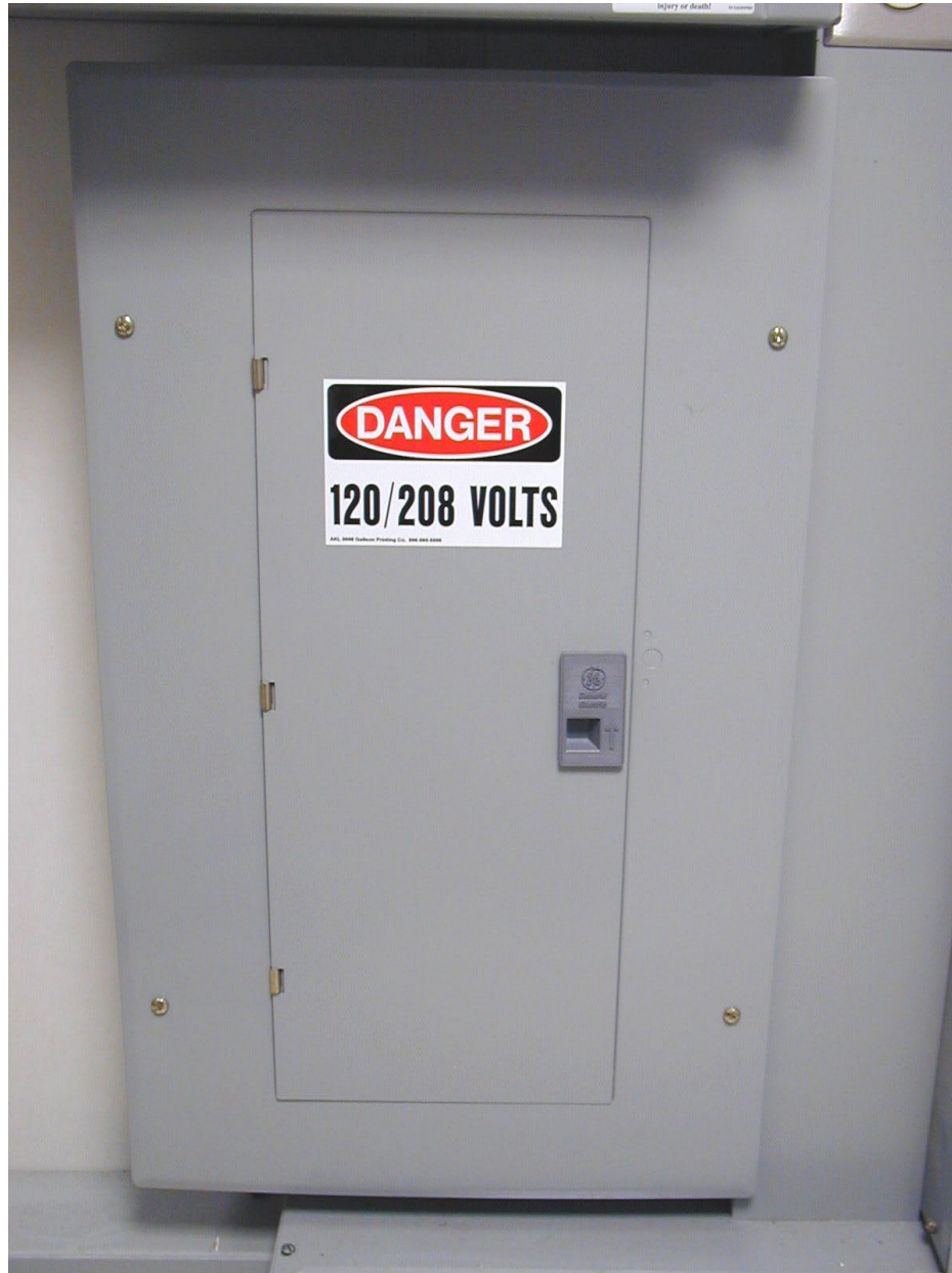
Figure 34: 120/208V AC Electrical Panel
