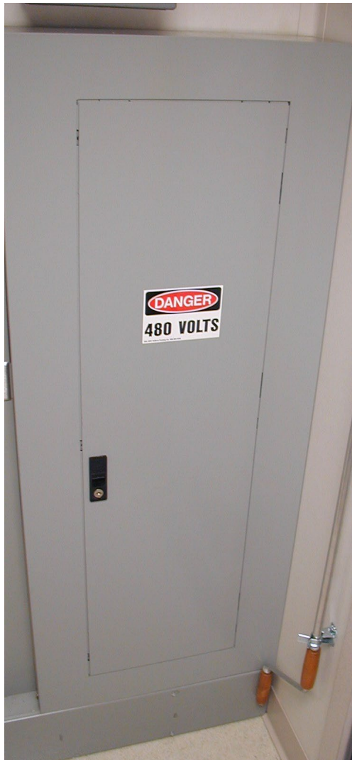
Figure 35: 480V AC Electrical Panel
