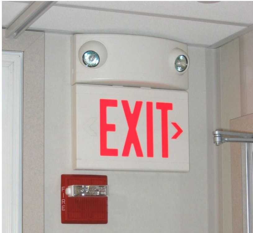
Figure 52: Emergency Dual Beam Lighting
