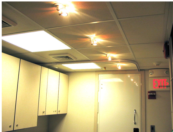
Figure 57: Control Room Lighting
