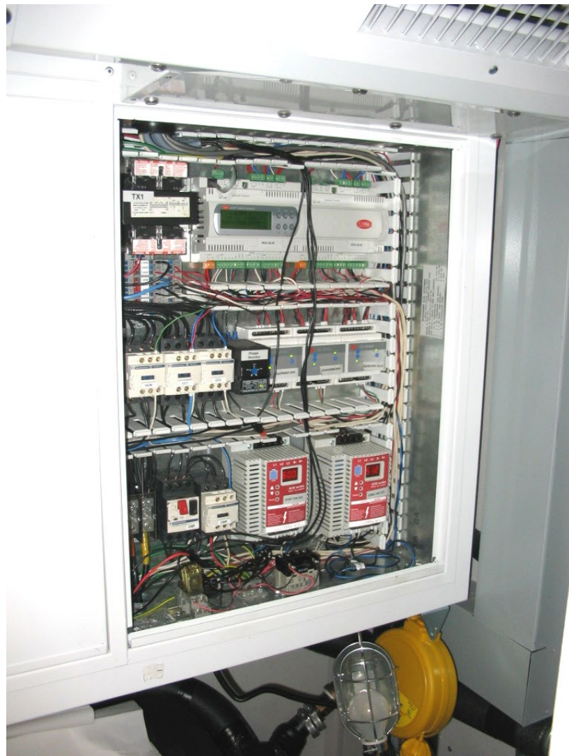
Figure 41: A/C / Chiller Control Panel
