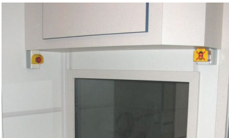
Scan Room E-Stop and Magnet Quench Controls
