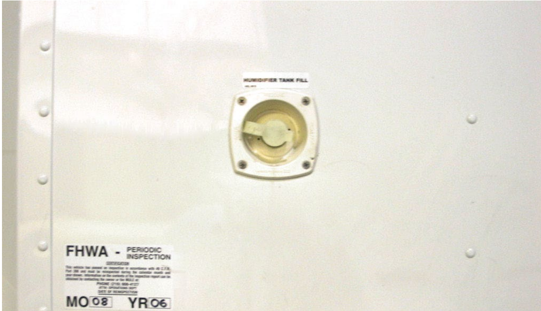
Figure 20: Fresh Water Connection
