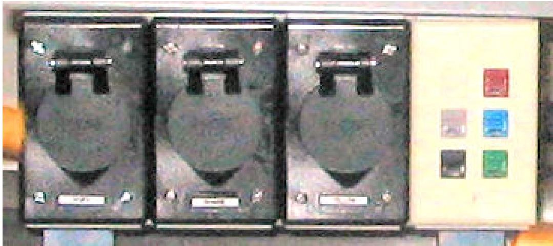
Figure 15: Phone & Data Line Connections
