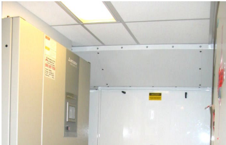
Figure 56: Equipment Room Lighting
