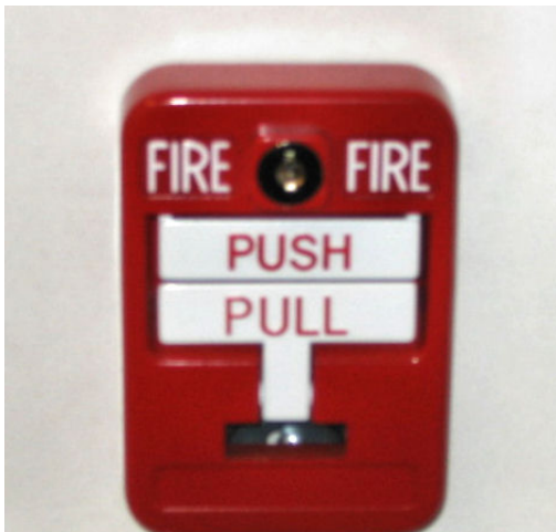
Figure 27: Fire Alarm Pull Station
