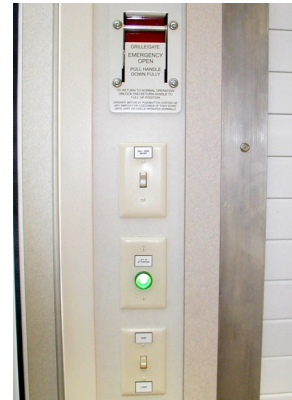
Roll Door Controls and Platform Lift "UP" light
