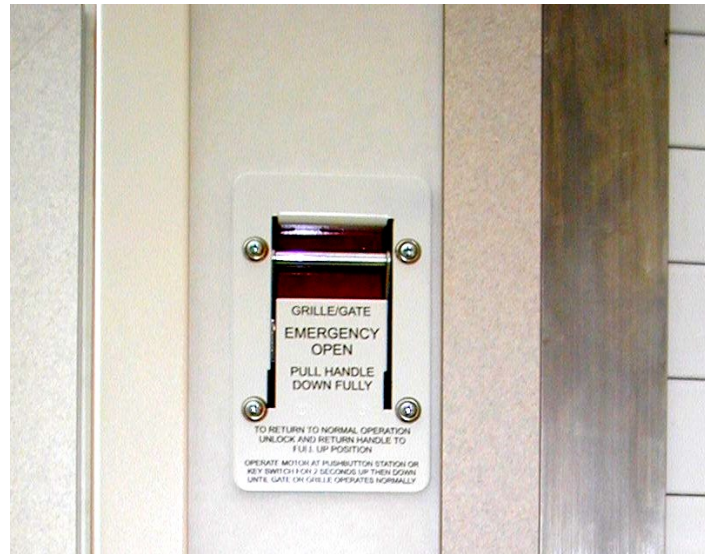
Figure 32: Roll Door Emergency Release
