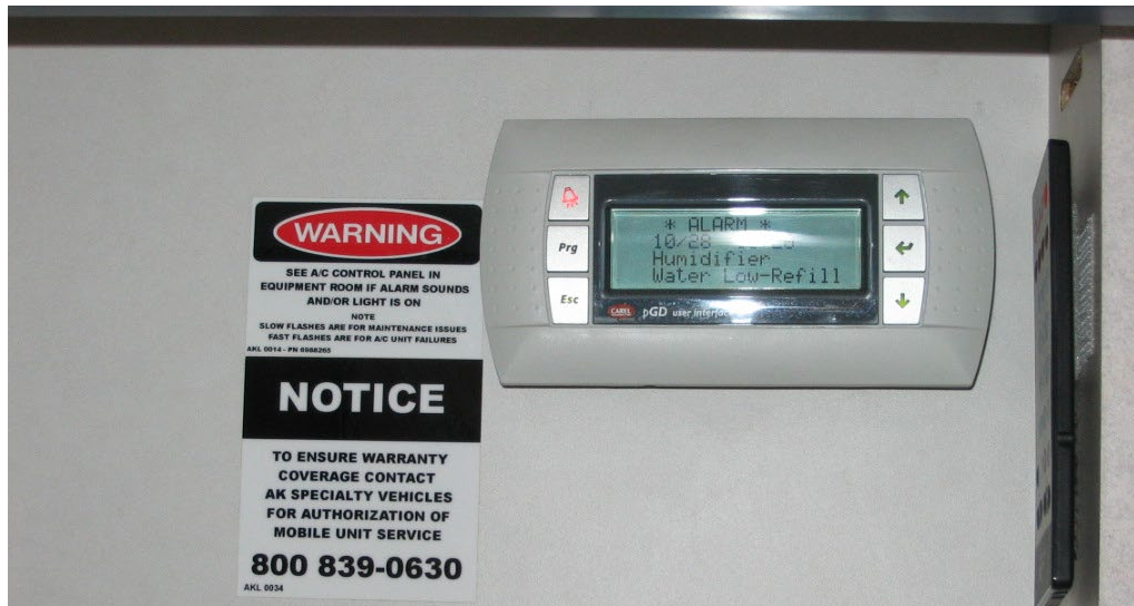
Figure 42: A/C / Chiller Alarm Panel
