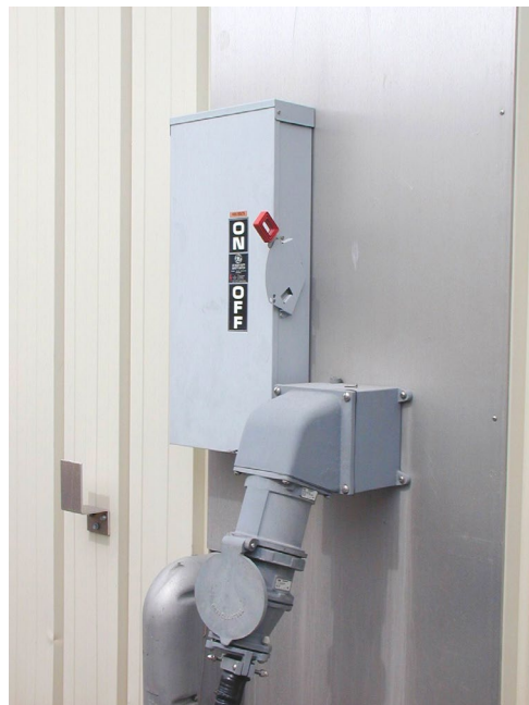
Figure 36: Shore Power Connection
