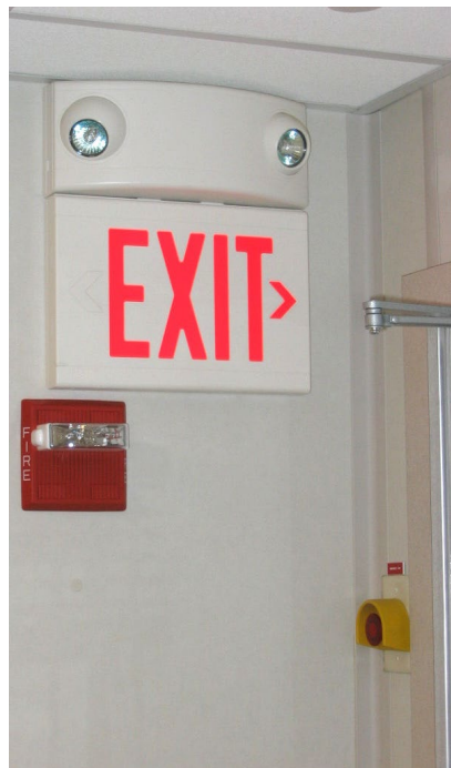
Emergency Off button, Control Room, next to Entry Door
