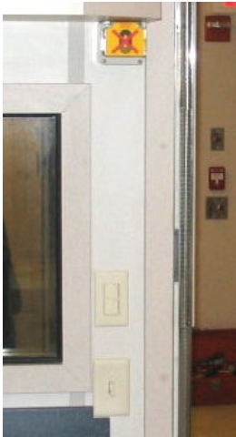
Scan Room Lighting and Magnet Quench Controls
