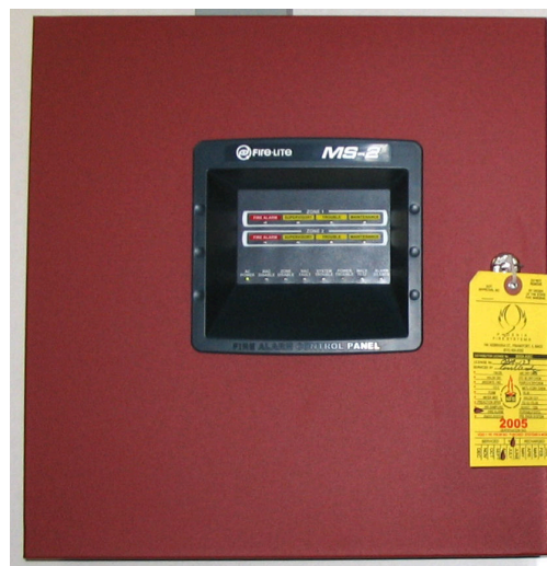
Figure 26: Fire Alarm Control Panel
