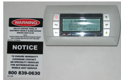
Air Conditioning Trouble Light & Alarm
