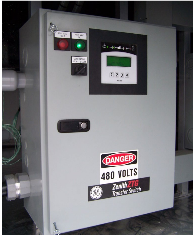
Figure 22: Automatic Transfer Switch and Phase Power Monitor
