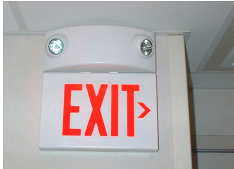
Control Room Emergency Light
