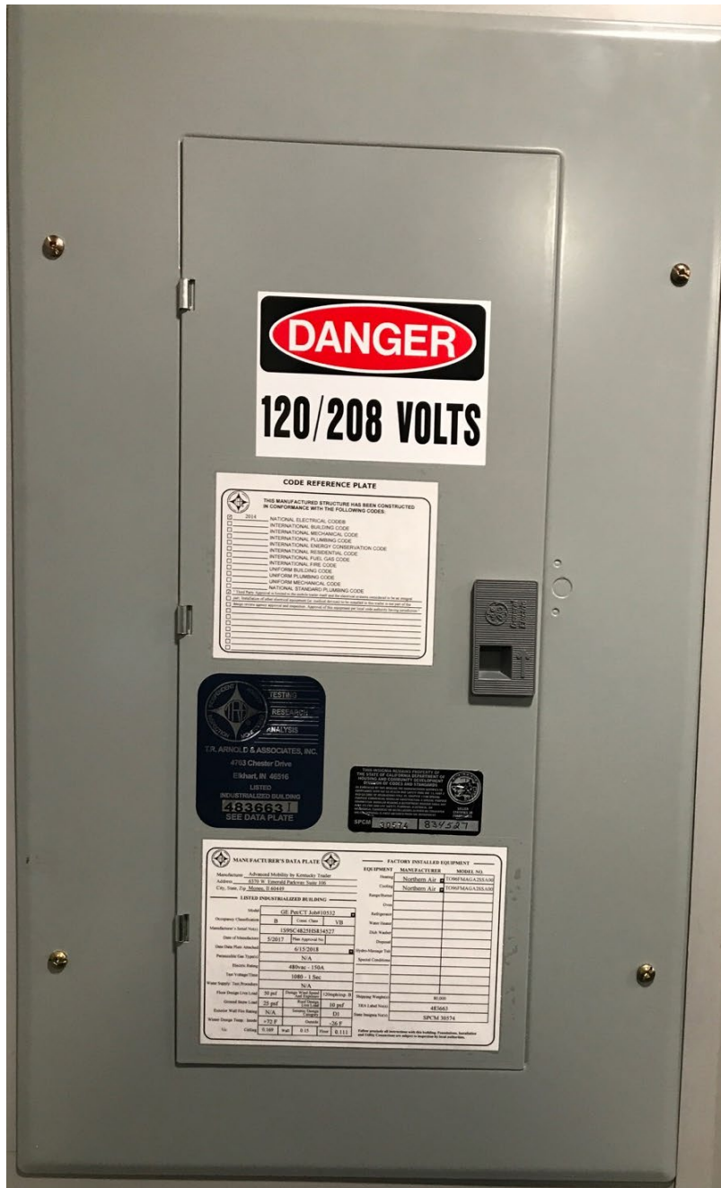
Figure 24: 120/208V AC Electrical Panel
