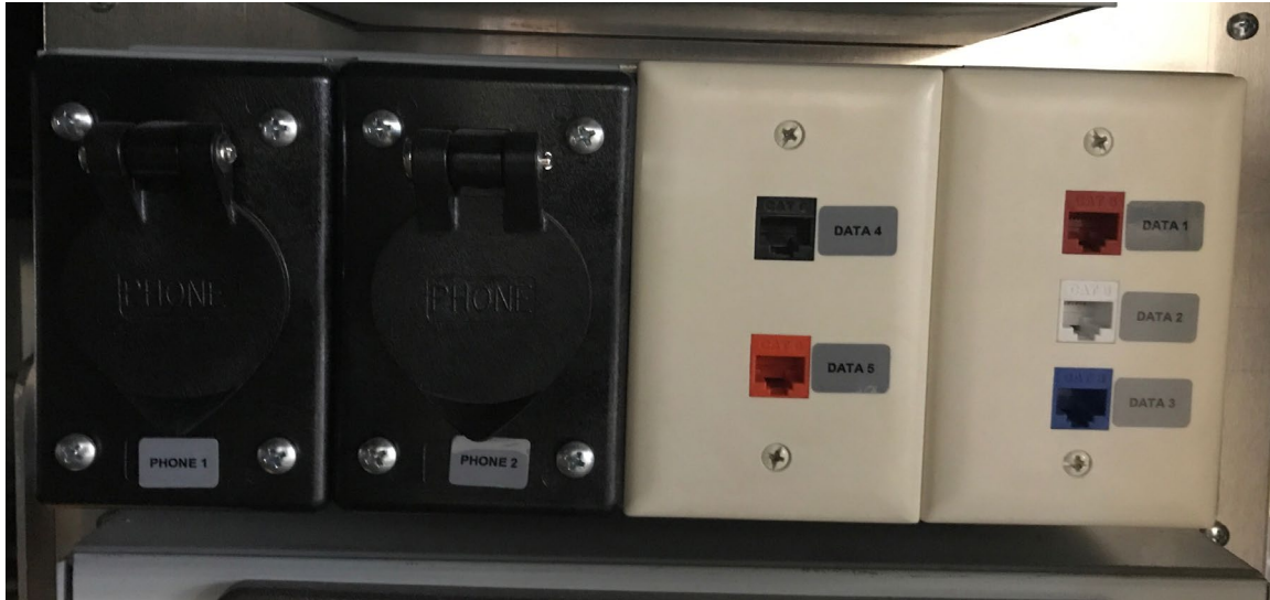
Figure 12: Phone & Data Line Connections
