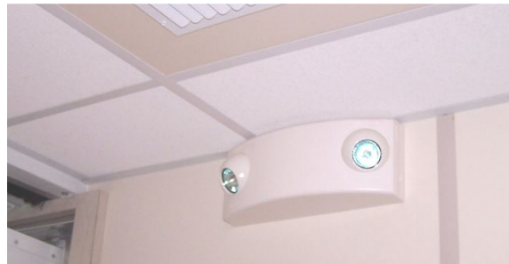
Gantry Room Emergency Light
