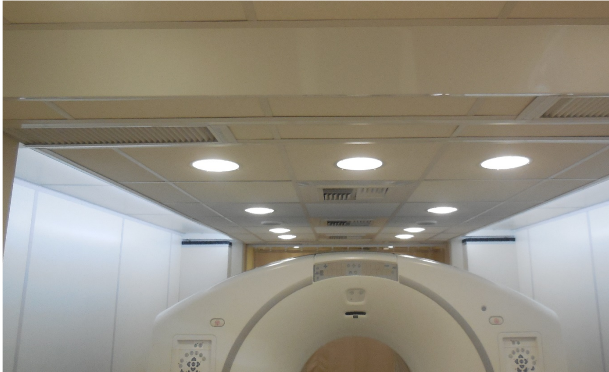
Figure 41: Gantry Room Overall Lighting
