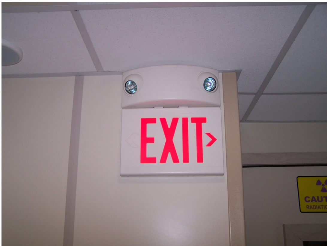
Figure 16: Control Room Emergency Lighting
