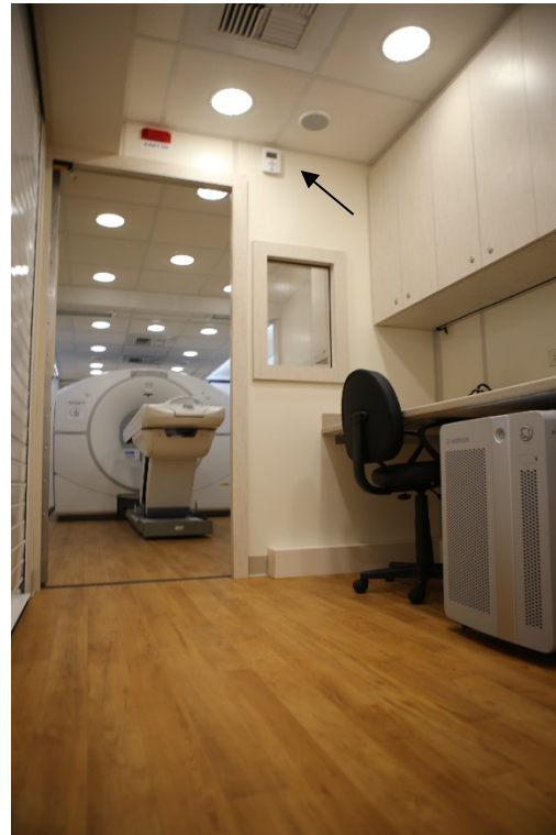
Control Room/Hot Lab Control
