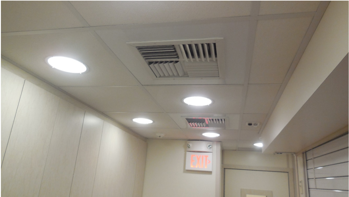
Figure 40: Control Room Overall Lighting
