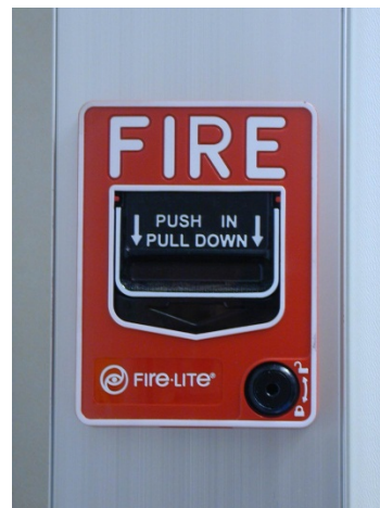
Figure 20: Fire Alarm Pull Station
