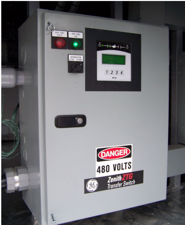
Figure 25: 480V AC ATS and Phase Power Monitor
